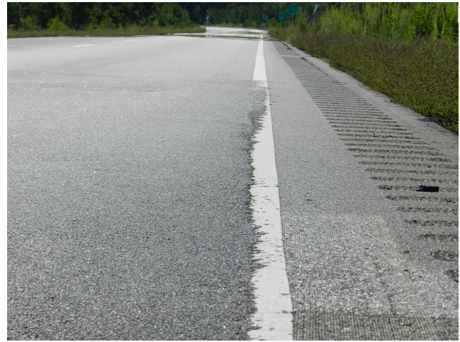
Figure 13. Degraded Lane Marking
