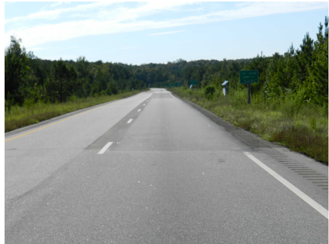
Figure 10. Missing Lane Markings
