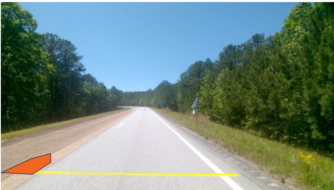
FIGURE 17 Subsection N13-B ARGG, 0.35-inch rutting, 3.1% cracking (April 2024).
