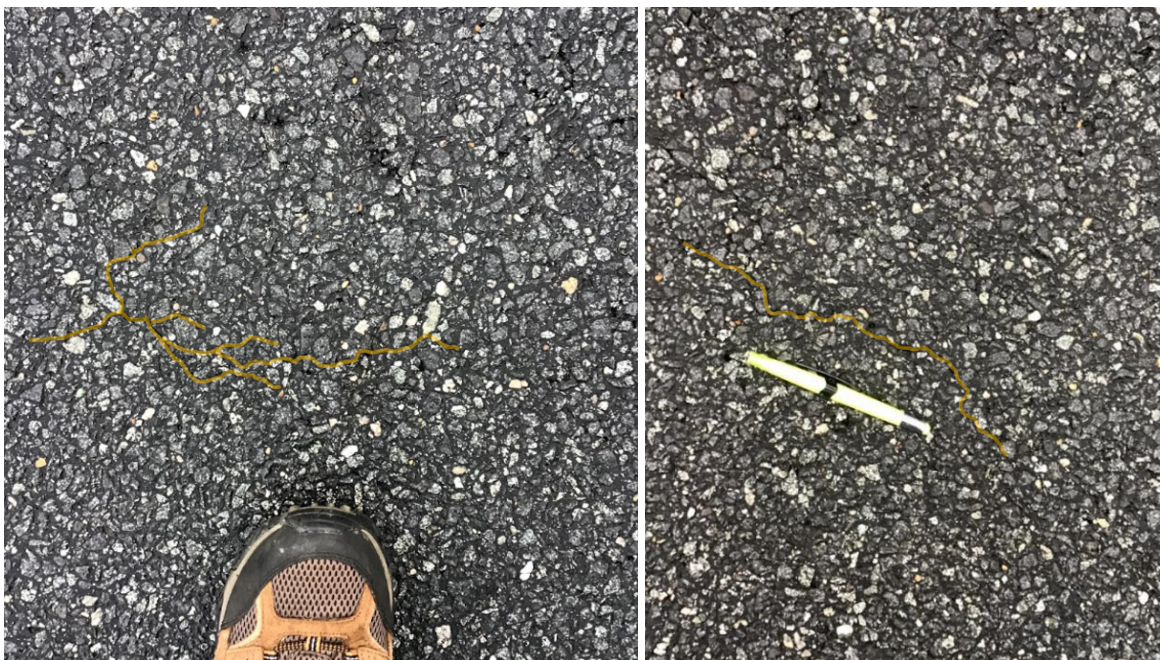
FIGURE 2 Sample cracking in N4 on 1/25/2021 (29.6 million ESALs).
