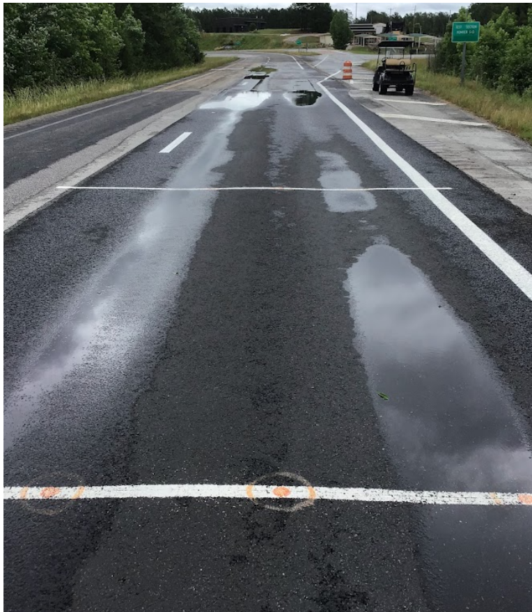
FIGURE 6 Rutting in Section S12 (April 2022).
