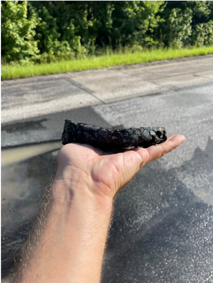
FIGURE 11 A core sample of the SMA layer in the transition zone at the end of the Section.
