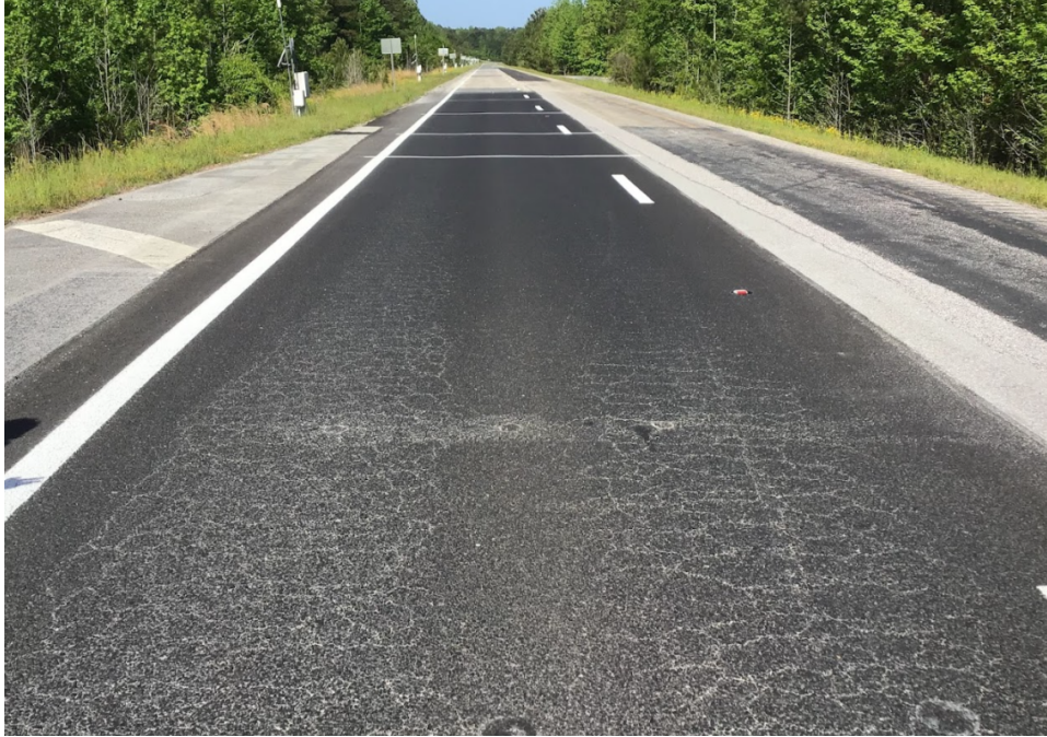
FIGURE 5 Cracking in Section S12 at approximately 1.3 million ESALs (April 2022).
