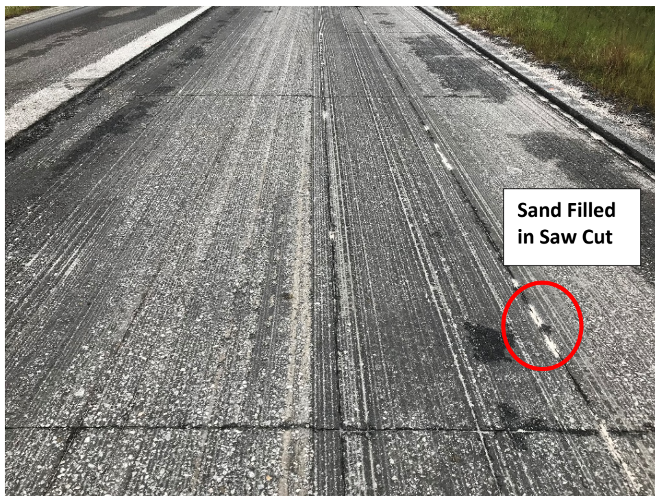
FIGURE 1 Deep saw cuts to simulate pavement cracks.
