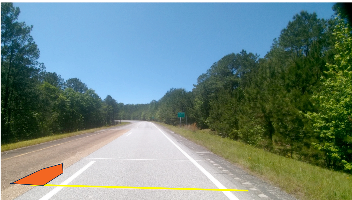
FIGURE 18 Subsection N13-B OGI, 0.19-inch rutting, 0.8% cracking (April 2024).
