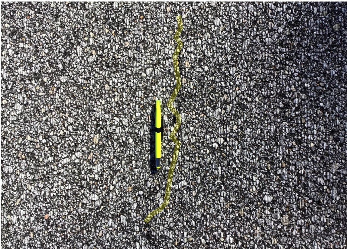
FIGURE 4 Longitudinal crack at edge of inside wheelpath in S9 at end of first test cycle.
