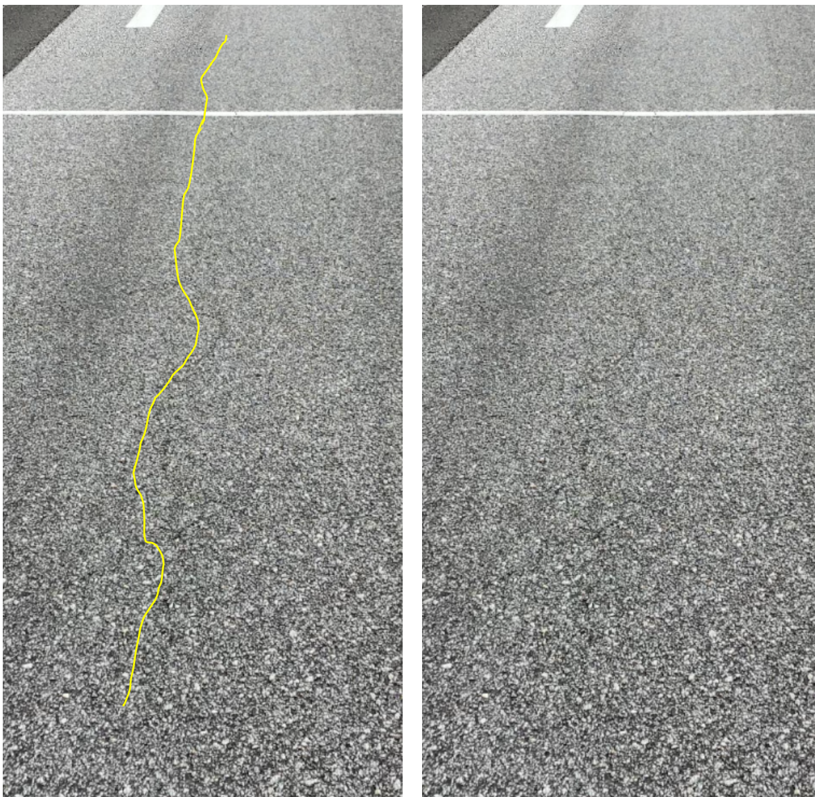
FIGURE 6 Longitudinal crack at edge of inside wheelpath in S9 at end of second test cycle (with and without highlighting).
