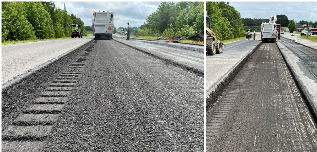
FIGURE 2 SMA and dense graded asphalt layer milling (left) and CCPR layer milling (right).
