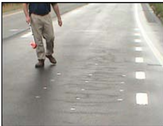
Figure 4. Progressed fatigue cracking
