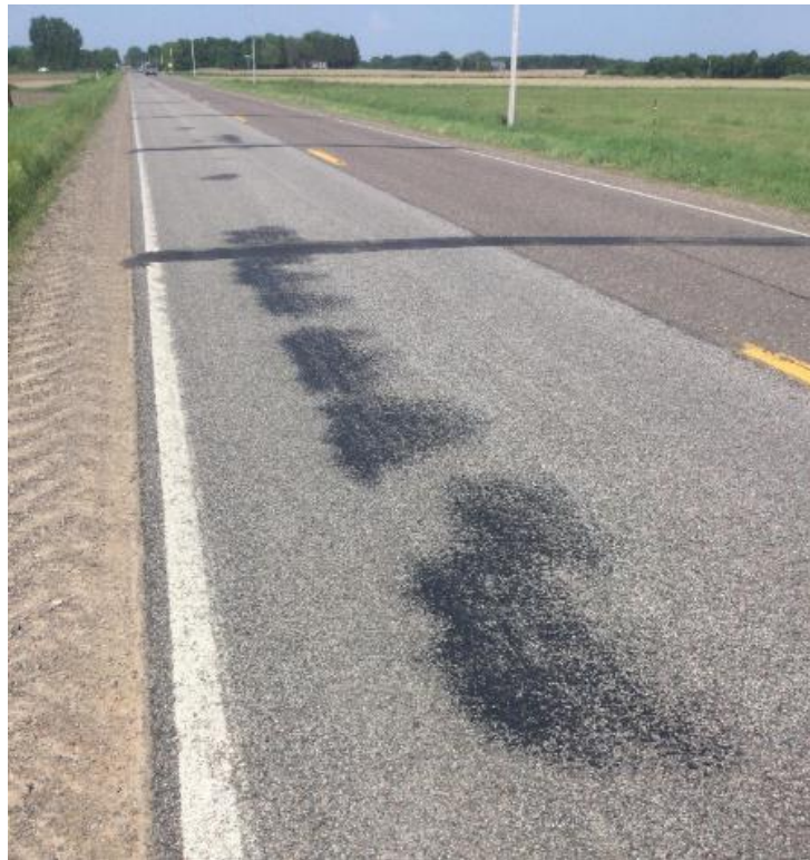
Figure 21. Isolated flushing in CSAH-8 at year 6.
