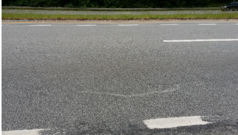
Figure 2. Cracking in US-280 sections.
