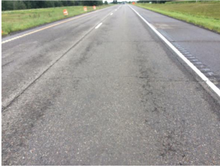
Figure 4. Overall pavement condition of US-169.
