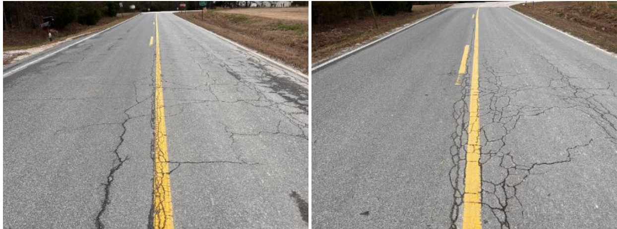
(a) 50% RAP thinlay (b) 5% RAS thinlay Figure 31. LR-159 high recycled content thinlay sections after 11 years.
