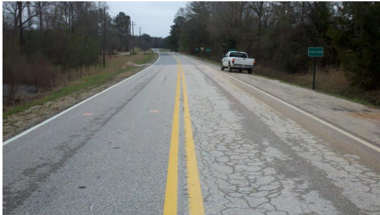
Figure 1. Variation in surface condition by lane in untreated pavement.
