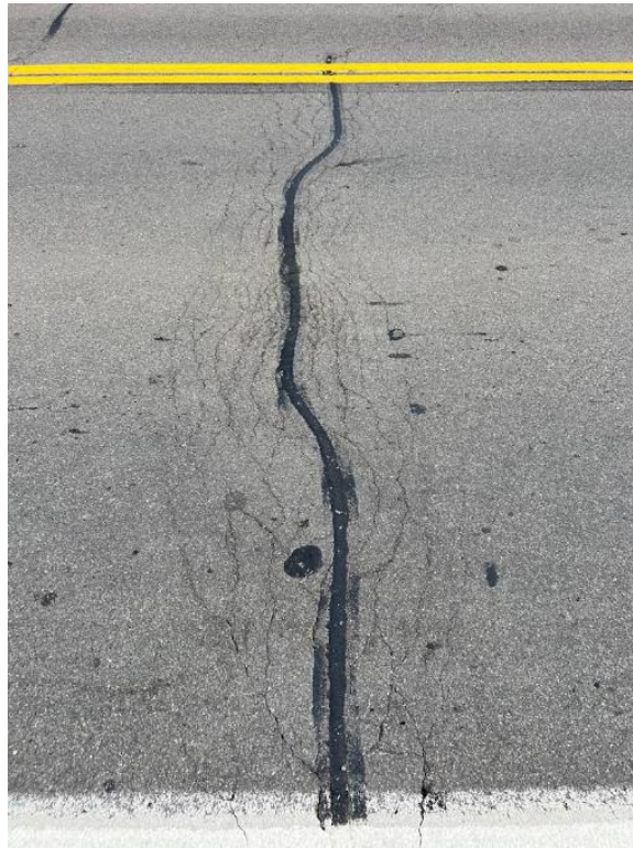
Figure 50. Transverse cracking in 70 th Street test section.
