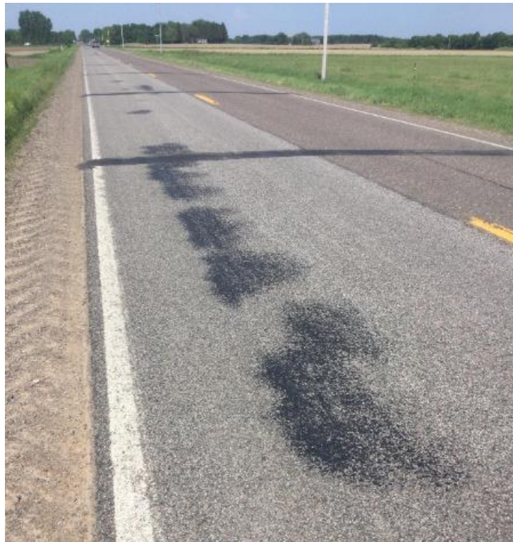
Figure 21. Isolated flushing in CSAH-8 at year 6.
