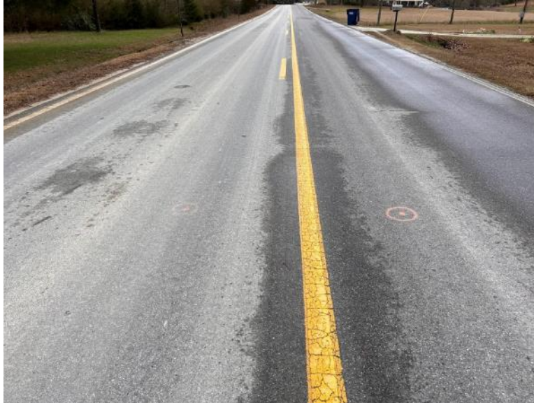
Figure 40. Scrub cape seal on LR-159 after 11 years of service.
