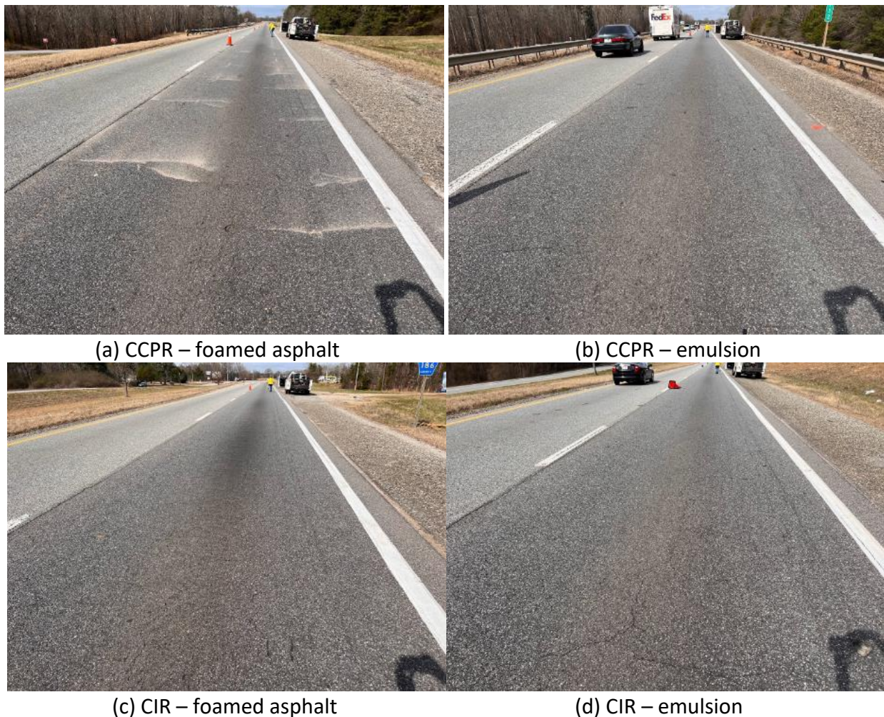
Figure 48. Overall condition of US-280 cold recycled sections after 7 years.
