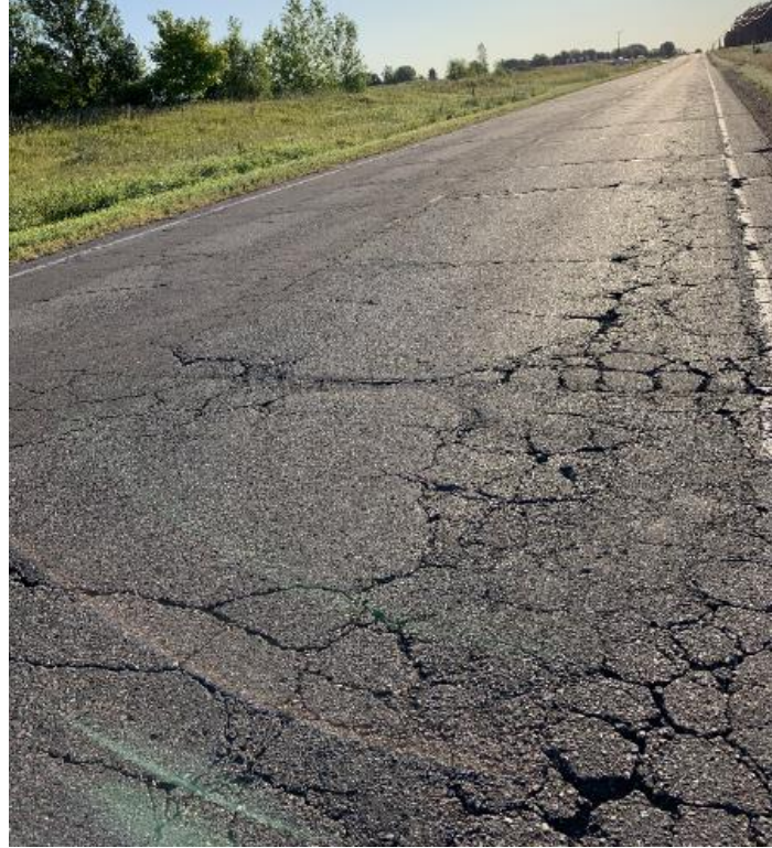
Figure 5. Overall pavement condition of 70 th Street.
