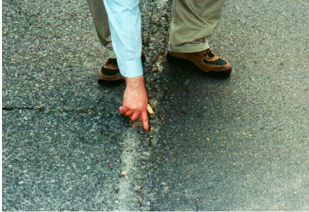
Figure 4. Close Up of Hwy 78 Cracking
