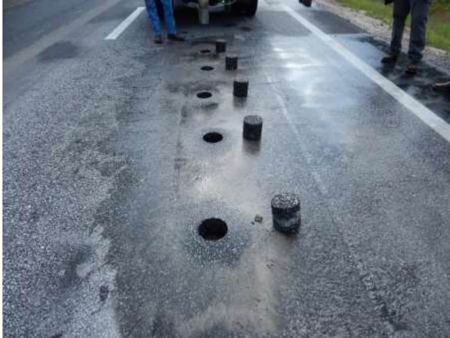
Figure 9. Cores Extracted in Section S8 in Distress Area (June 2022).
