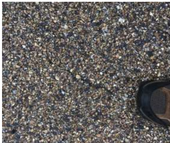
FIGURE 5 Minor between-wheelpath longitudinal cracking in S2.
