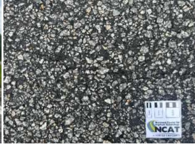
E6A (87.8% of G_{mm} ) representative cracking
