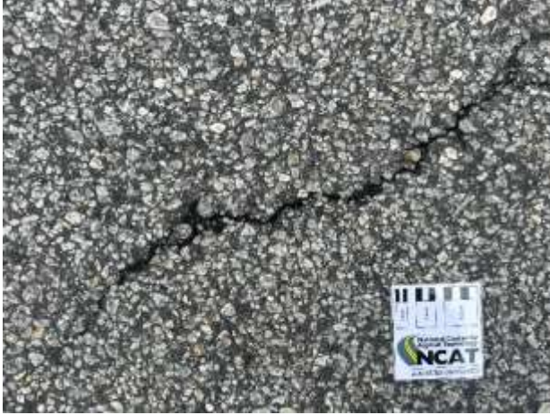
E5A (93.6% of G_{mm} ) representative cracking
