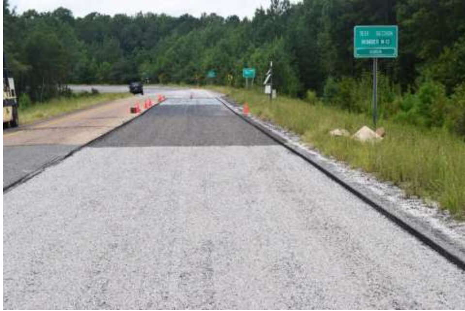
FIGURE 3 Section N12-C chip seal with No. 7 stone (foreground) and N13-A chip seal with RAP (background).
