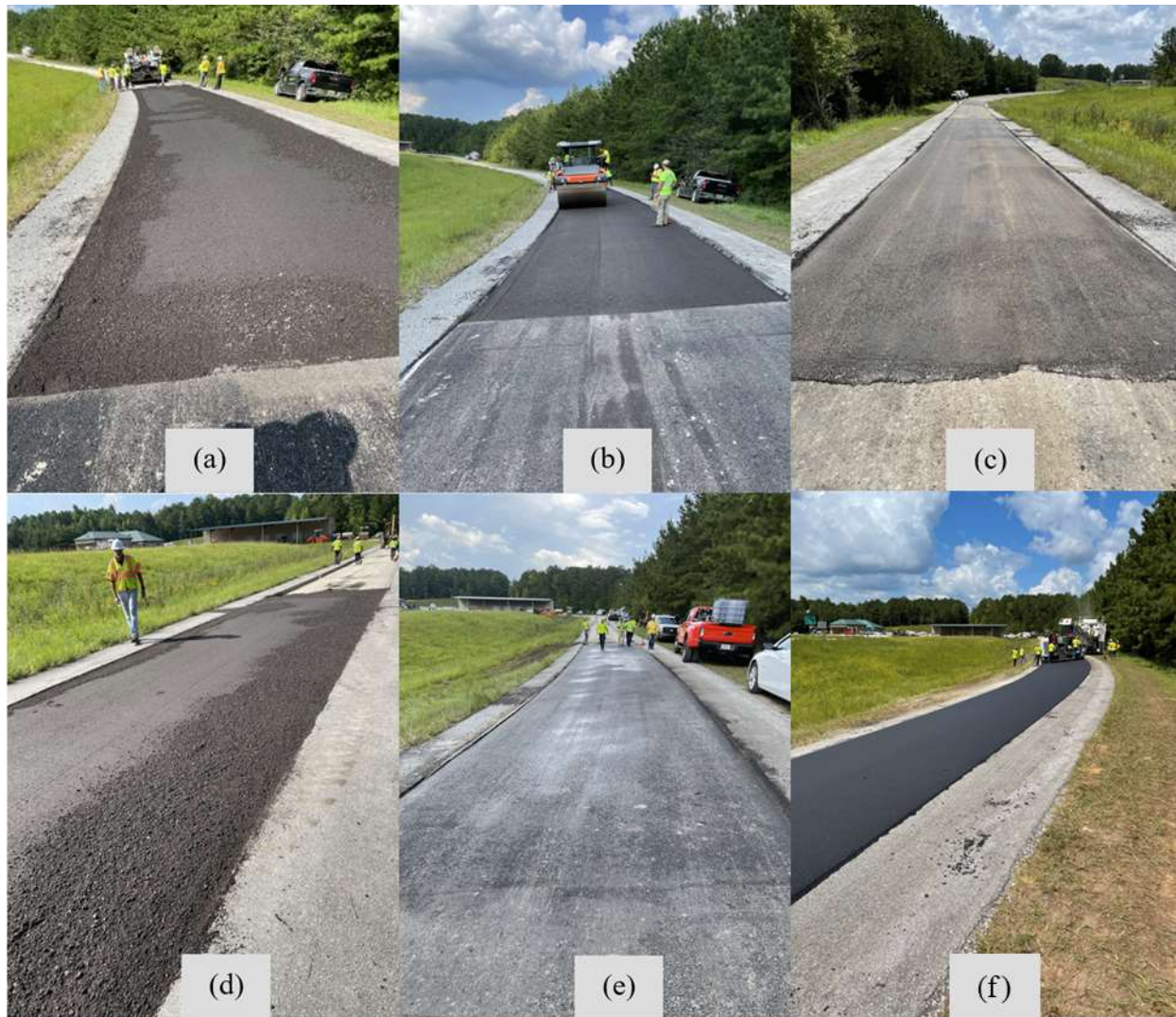
FIGURE 4 Paved CCPR Sections on off-ramp; (a) foamed asphalt with active filler, (b) engineered emulsion, (c) CR rejuvenator, (d) emulsified bio-based rejuvenator; (e) emulsified bio-based rejuvenator, and (f) HMA thinlay overlay.
