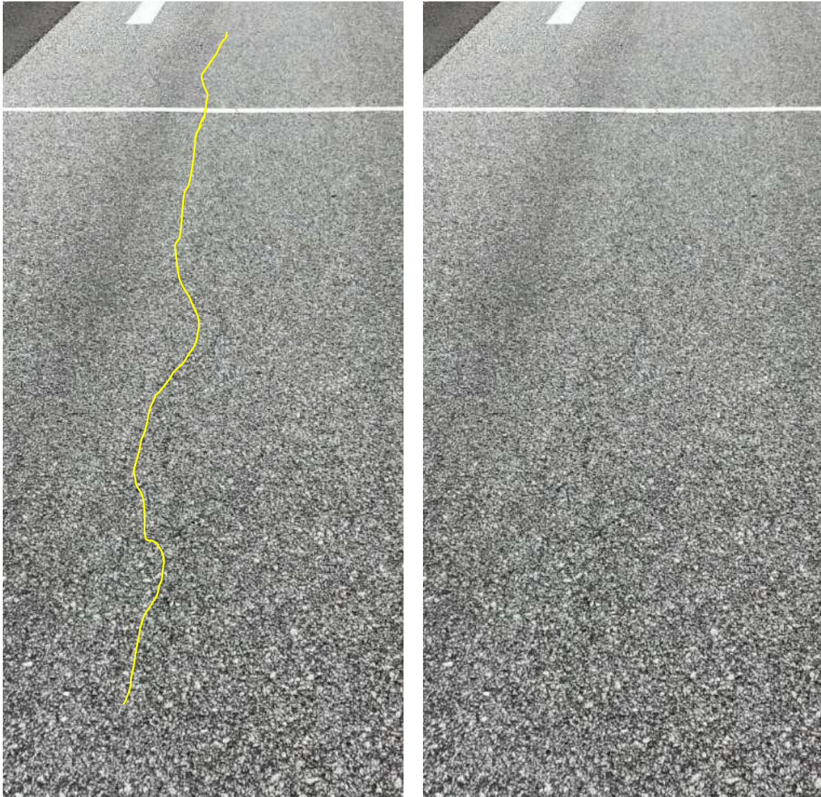
FIGURE 6 Longitudinal crack at edge of inside wheelpath in S9 at end of second test cycle (with and without highlighting).
