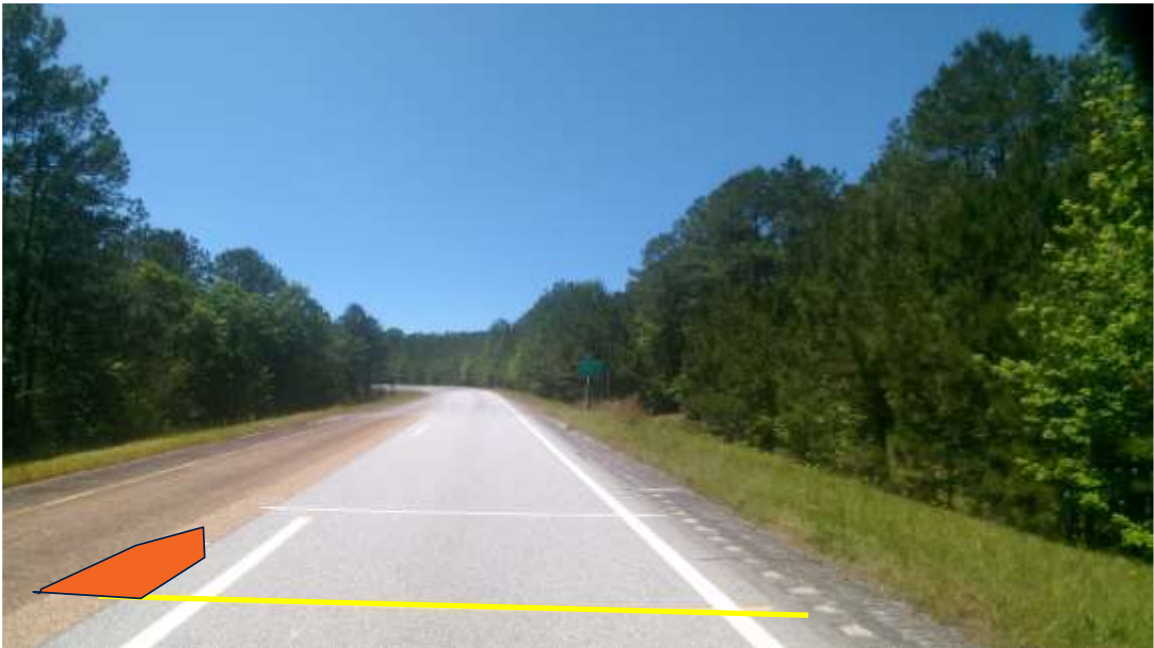
FIGURE 18 Subsection N13-B OGI, 0.19-inch rutting, 0.8% cracking (April 2024).
