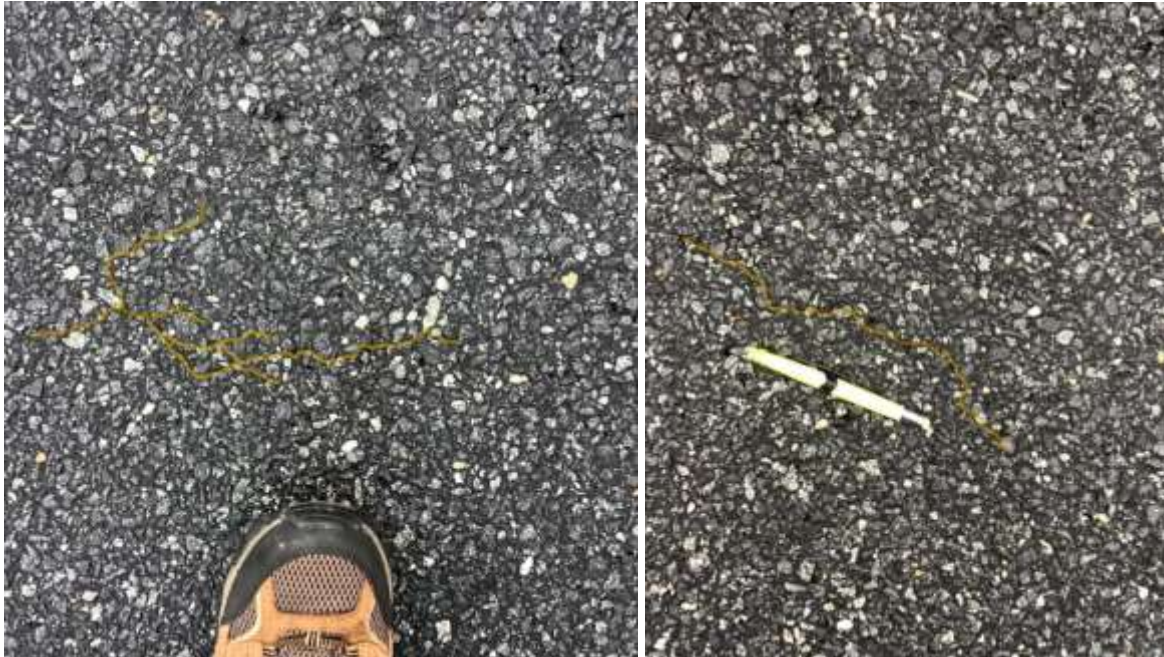
FIGURE 2 Sample cracking in N4 on 1/25/2021 (29.6 million ESALs).
