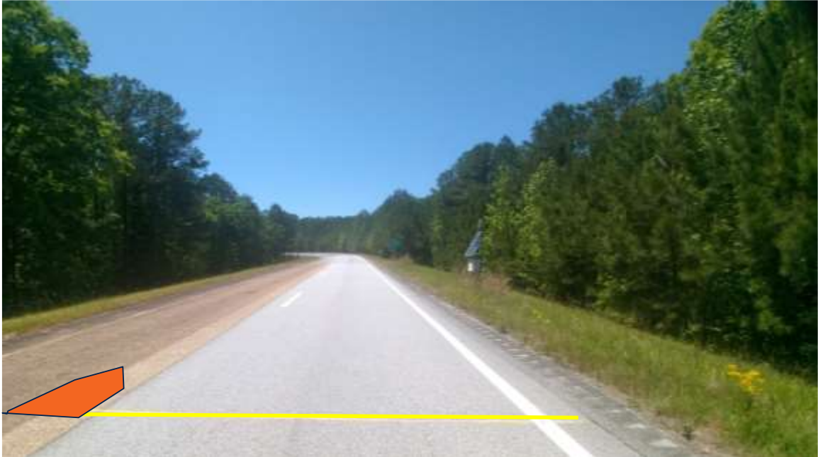
FIGURE 17 Subsection N13-B ARGG, 0.35-inch rutting, 3.1% cracking (April 2024).
