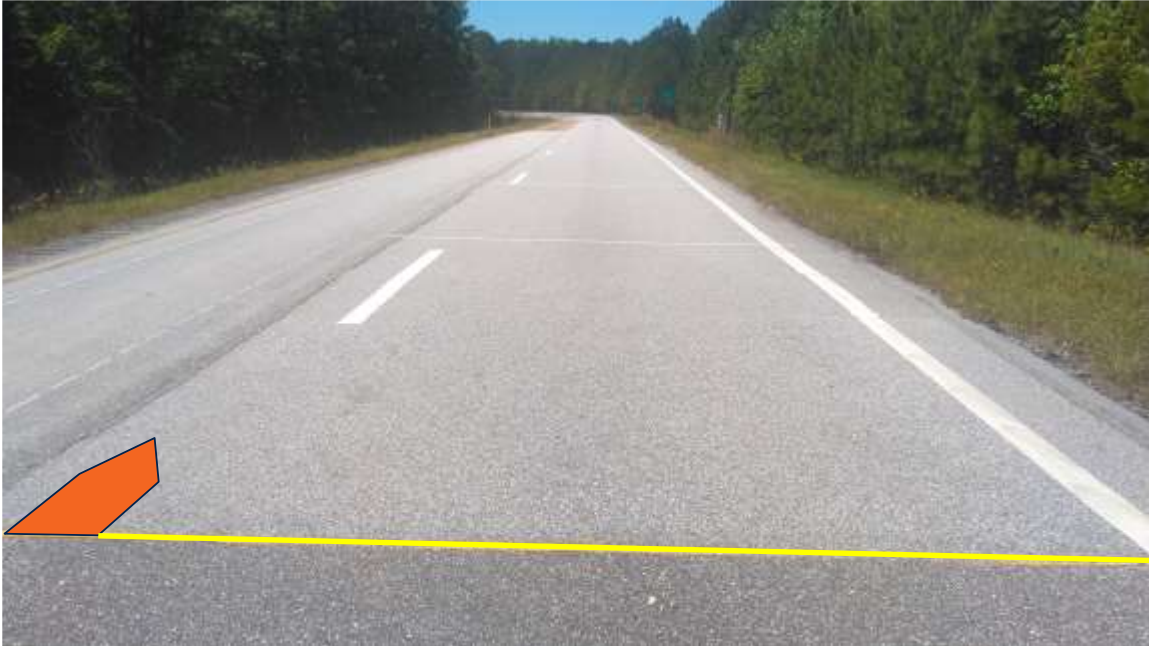
FIGURE 13 Subsection N12-A GlasGrid ® , 0.24-inch rutting, no cracking (April 2024).
