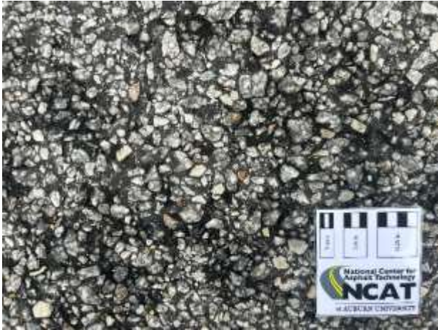
E5B (92.0% of G_{mm} ) representative cracking
