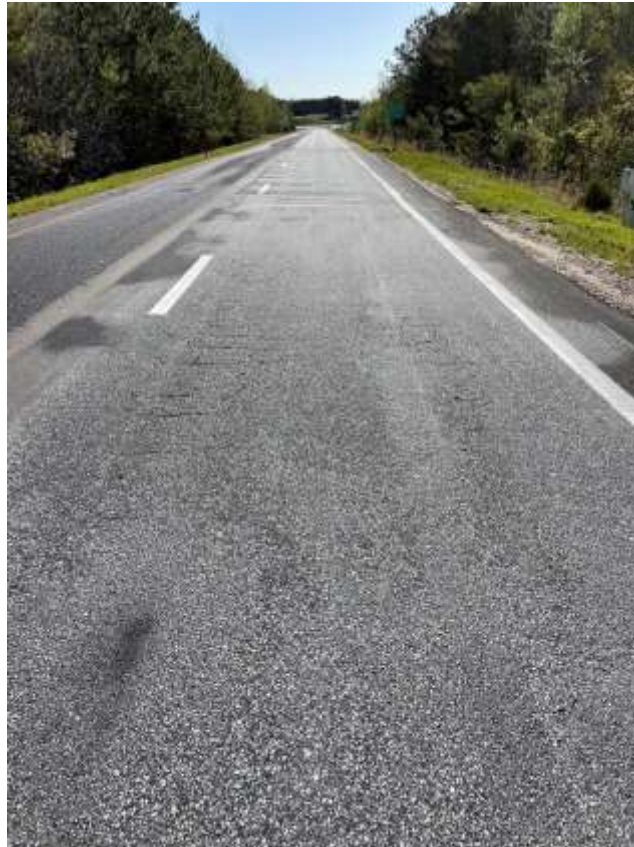
Figure 8. Cracking in Section S8 at approximately 1.2 million ESALs (April 2022).
