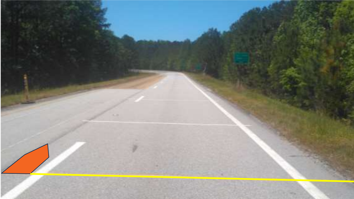
FIGURE 15 Subsection N12-C virgin chip seal, 0.21-inch rutting, no cracking (April 2024).
