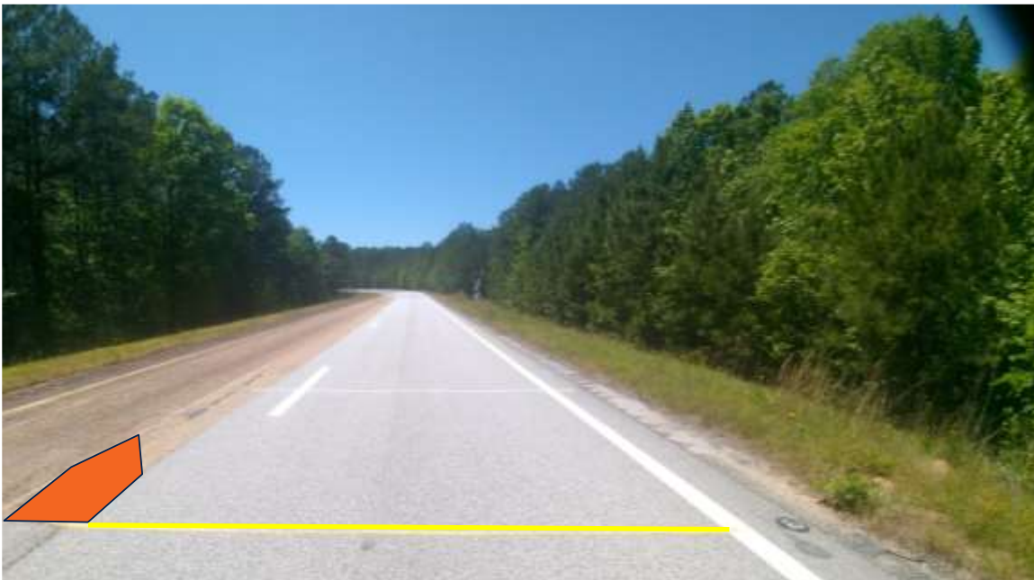
FIGURE 16 Subsection N13-A RAP chip seal, 0.41-inch rutting, 0.8% cracking (April 2024).
