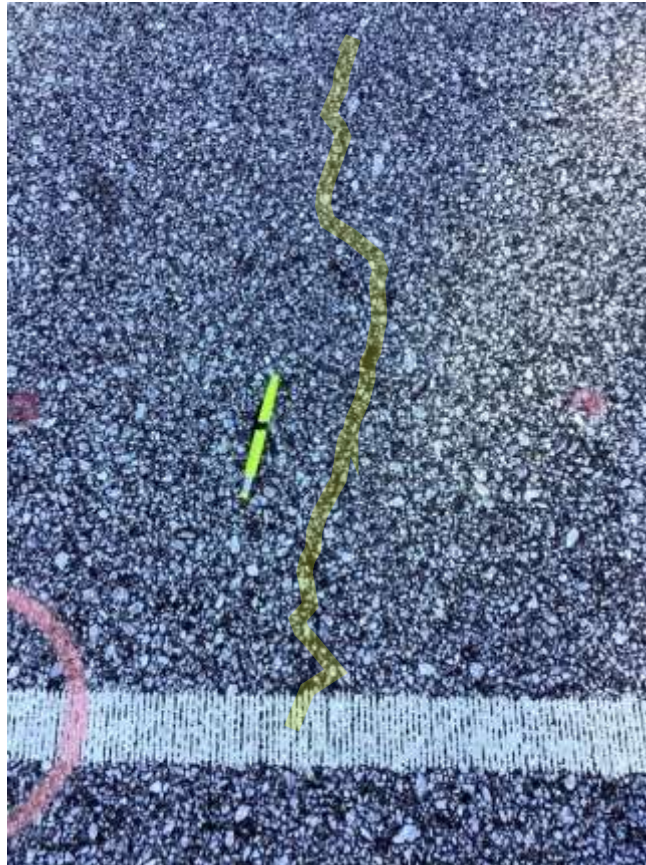
FIGURE 3 Longitudinal crack at edge of outside wheelpath in S9 at end of first test cycle.
