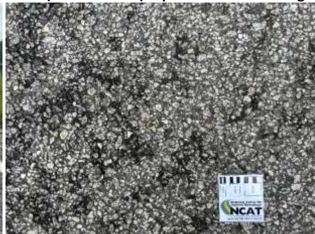
E6B (89.7% of G_{mm} ) representative cracking
