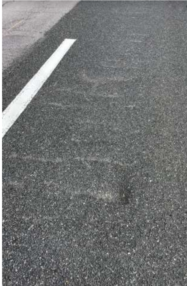
FIGURE 3 Wheelpath fatigue cracking in N4 on 1/22/2024 (39.1 million ESALs).
