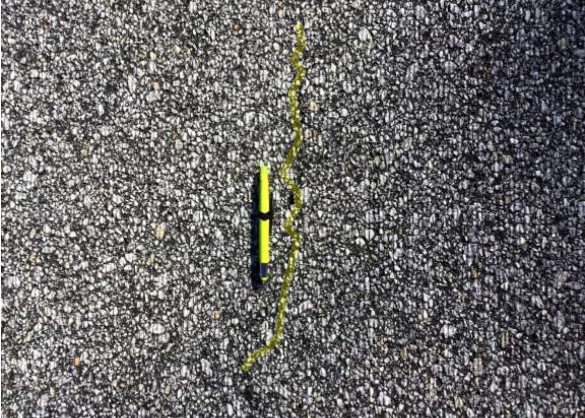
FIGURE 4 Longitudinal crack at edge of inside wheelpath in S9 at end of first test cycle.
