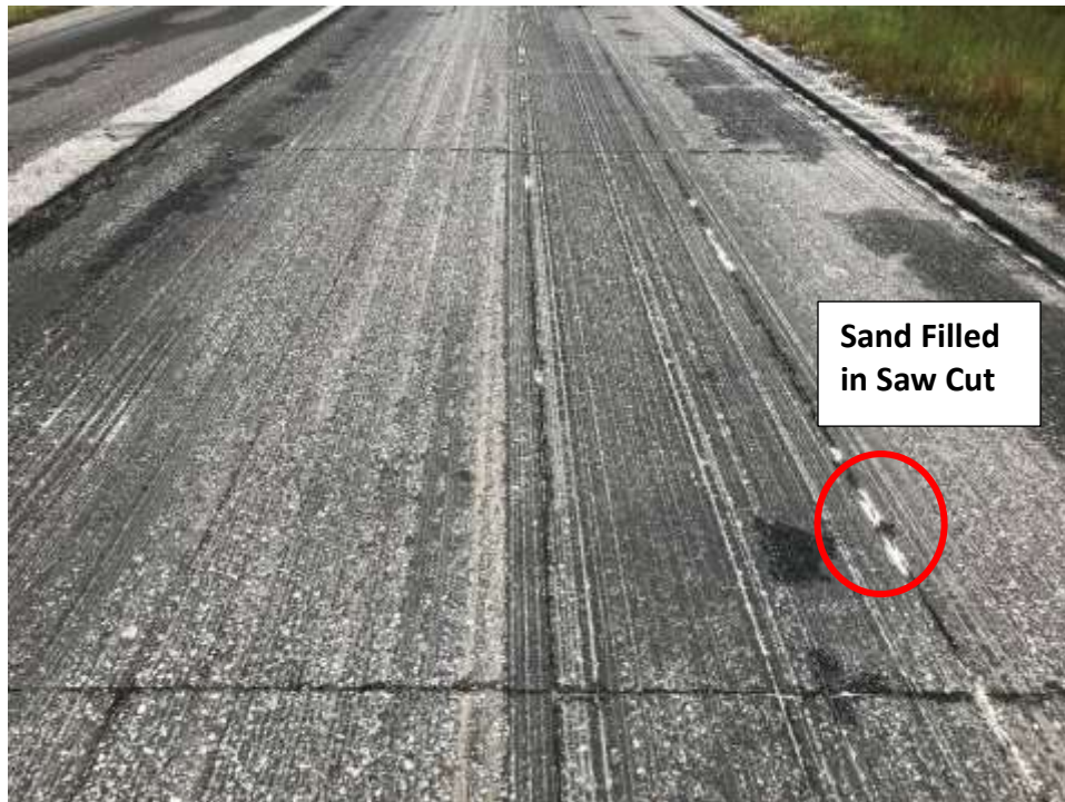
FIGURE 1 Deep saw cuts to simulate pavement cracks.
