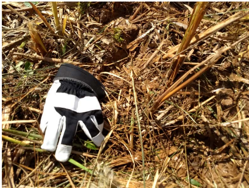
Figure 12 – Resulting bottom of the channel after clearing of channel vegetation. Soil was slightly covered with residual vegetation, and with high erosive potential
