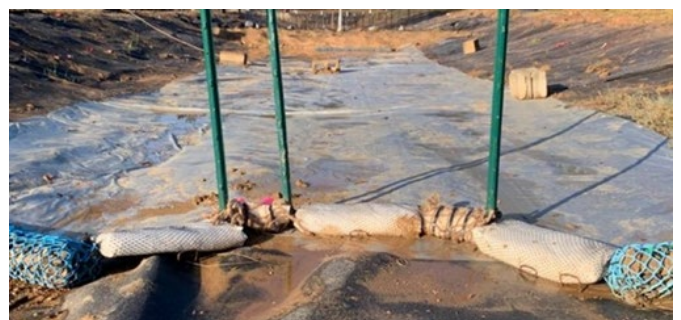
Flocculant blocks in inflow channel
