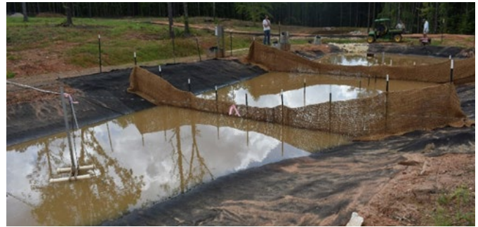
Lined basin with baffles
