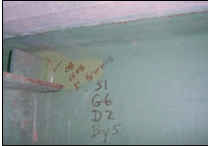
Figure 4.3 Fatigue cracks at upper end of the connection plate (Bowman et al. 2012)
