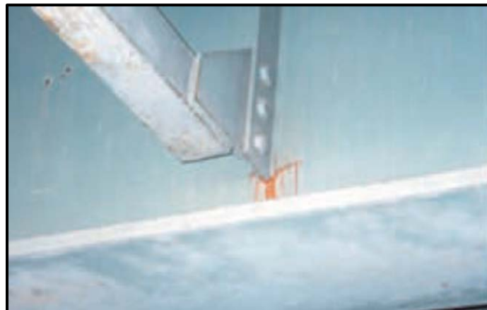
Figure 4.2 Fatigue cracks at lower end of the vertical connection plate (Bowman et al. 2012)
