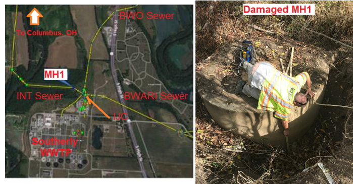
FIG. 1. Location of MH1 with respect to IJC and nearby sewer lines, and damage following 3/25 flow interruption
