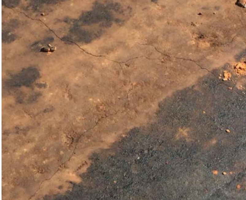
Figure 2.8: Shrinkage Cracks in Soil Cement (McLaughlin 2017)
