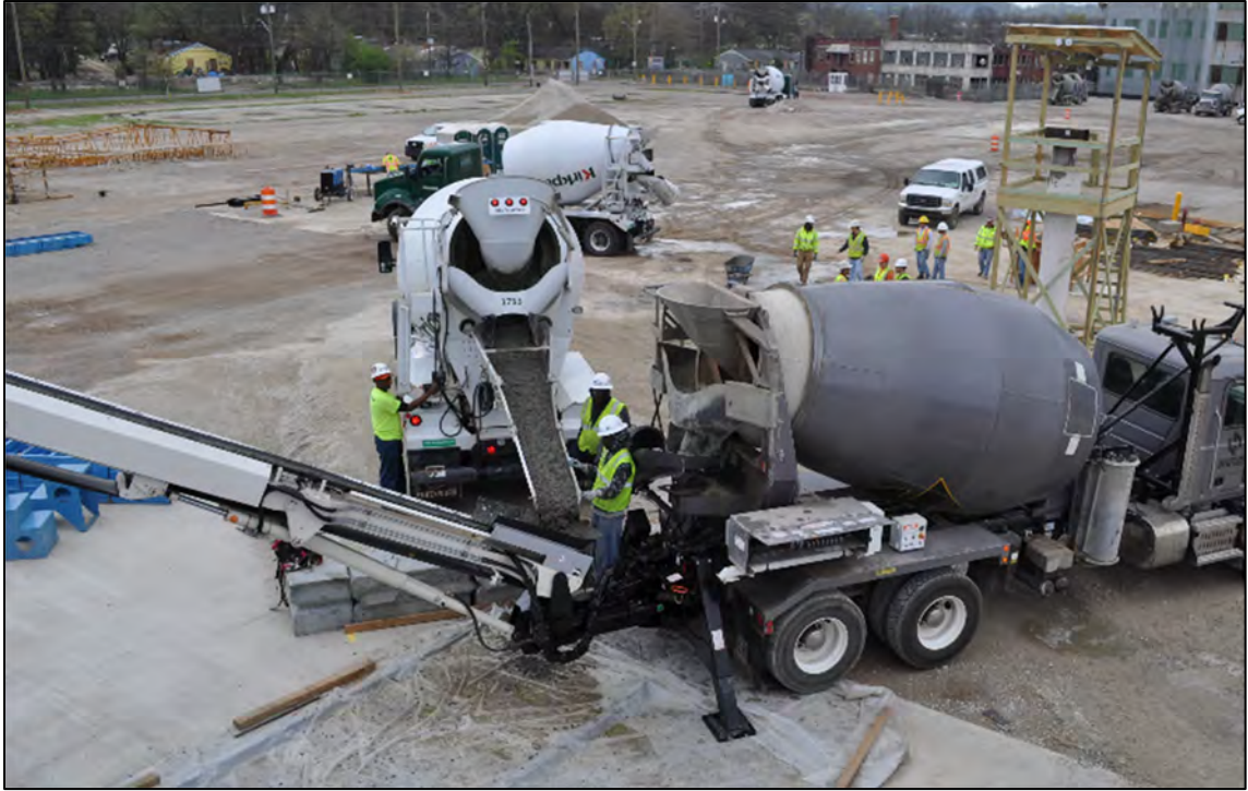
Figure 5-8: Conveyor moving concrete to desired location at the top of the formwork
