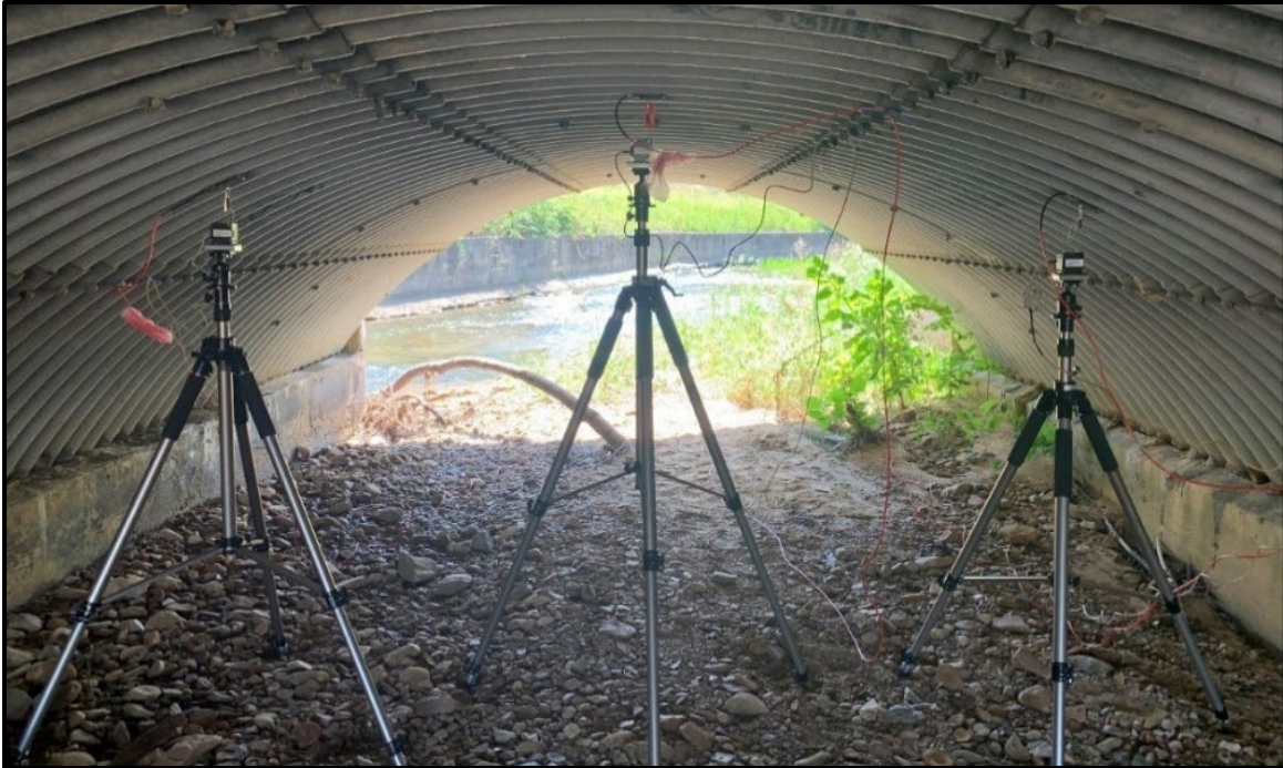
Figure 5.28. Potentiometers installed at 1/4, crown and 3/4 locations at Bain's Gap Road culvert.
