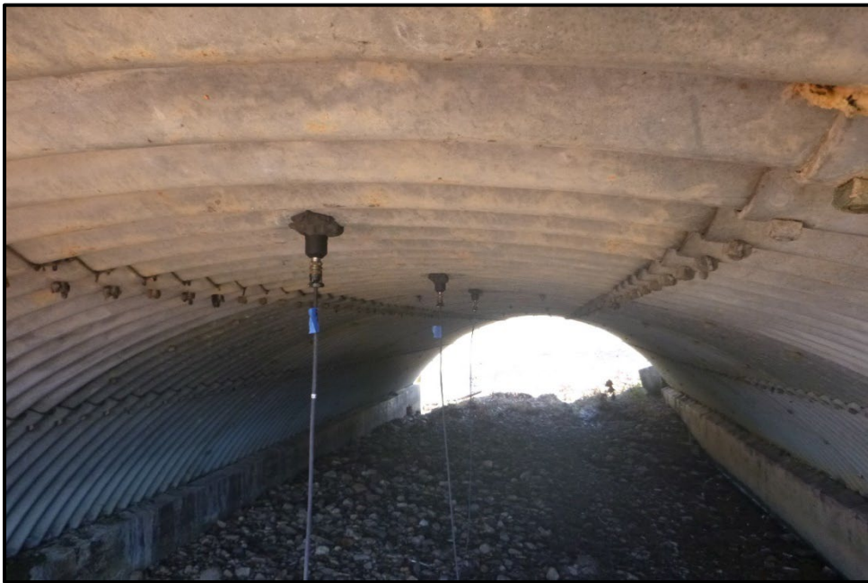
Figure 4.23. Accelerometers to measure wave transmission Lennox Avenue.
