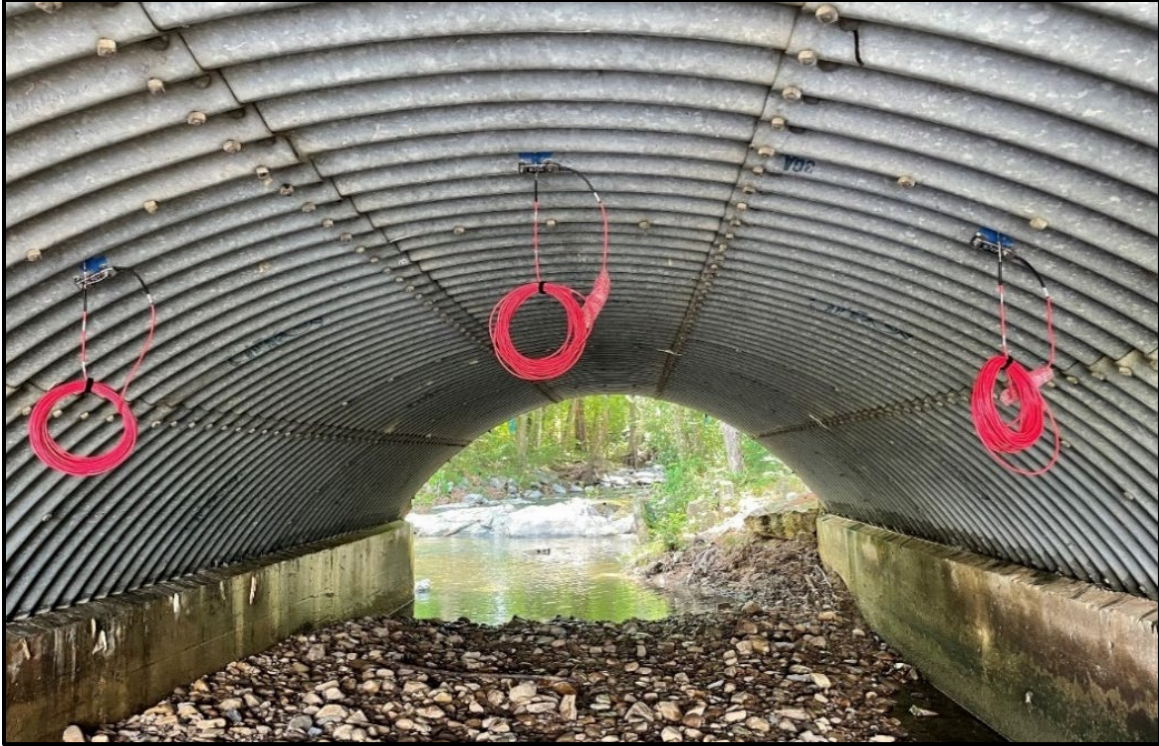
Figure 5.26. Strain gage installed at \frac{1}{4} , crown and \frac{3}{4} of the Berman Road culvert.
