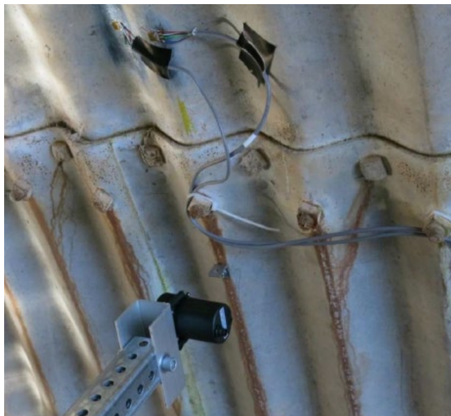
Figure 2.12. Close-up view of instrumentation point (Sargand et al. 2018).
