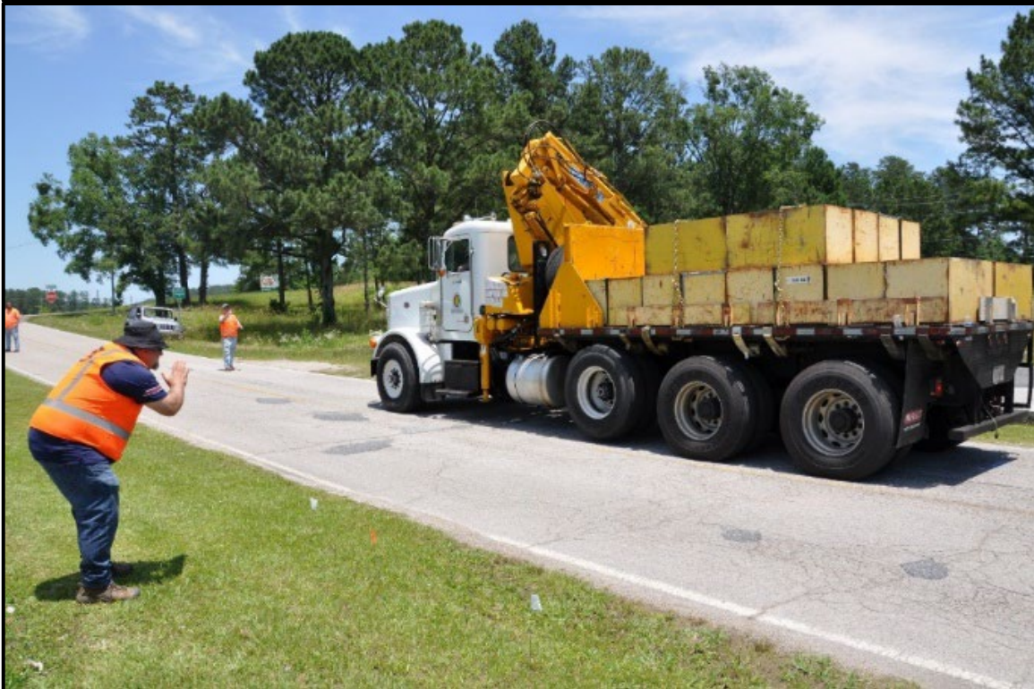
Figure 5.31. Verification of truck location in stopping point (load line 1) at the Bain’s Gap Road culvert.
