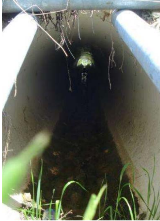
Figure 4-18: Water and Sediment Buildup within Pipe
