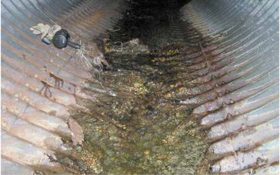
Figure 5-23: Corrosion of Corrugated Metal Culvert (Matthews et al. 2012)
