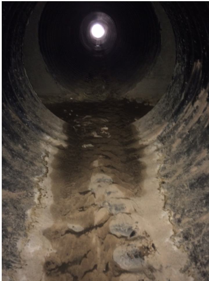
Figure 4-32: Sediment Collected in Bottom of Junction Box of Station 224+00 Pipeline
