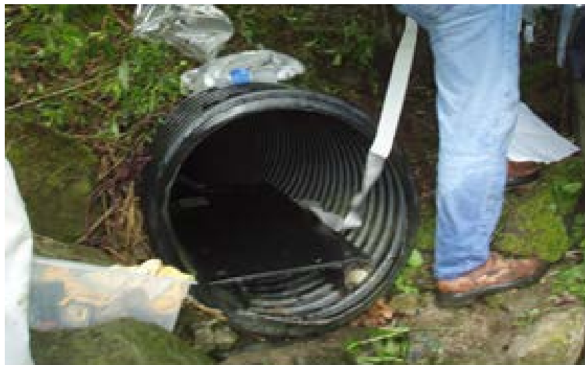
Figure 2-5: East End of Type C HDPE Pipe (Goddard 2008)
