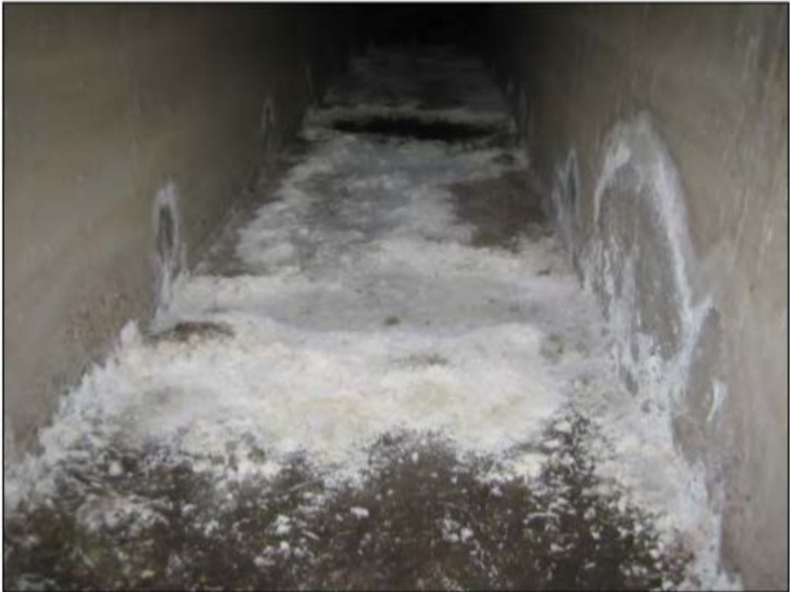
Figure 5-22: Corrosion of Reinforced Concrete Culvert (Molinas and Mommandi 2009)
