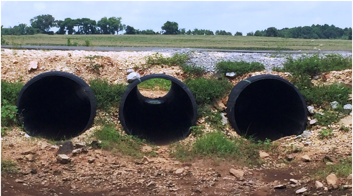
Figure 3-22: Colbert County HDPE Pipeline Front View
