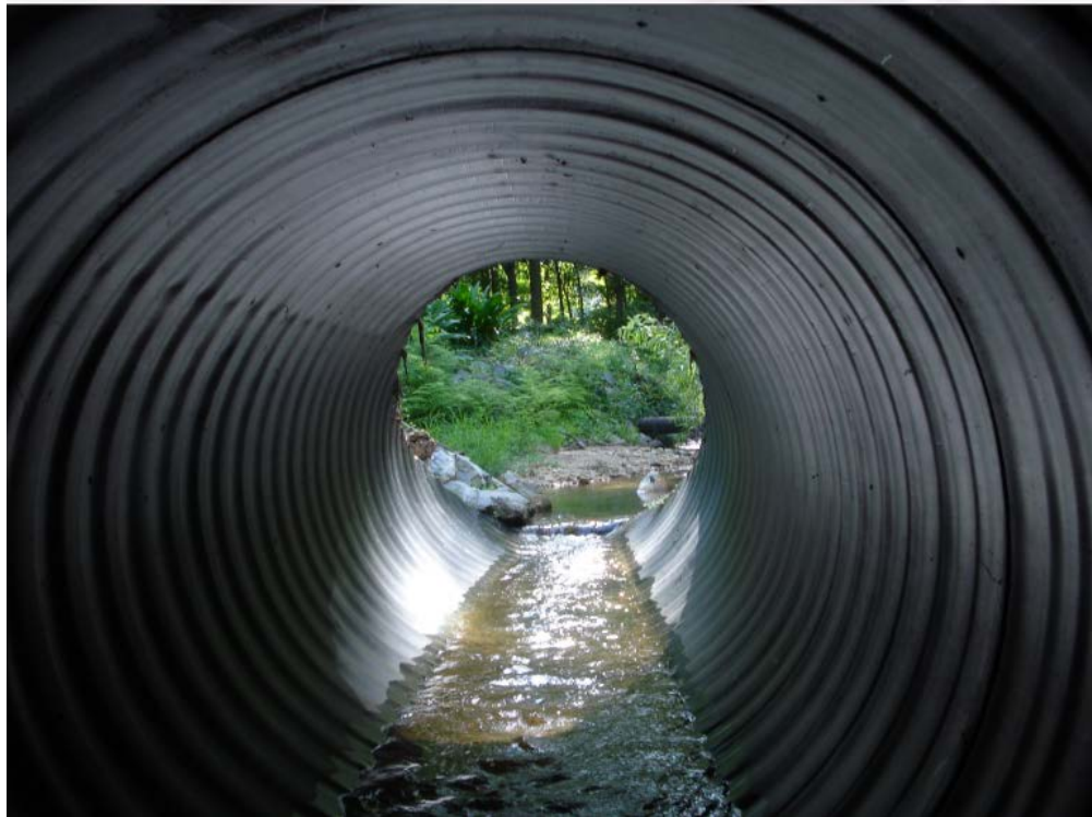
Figure 3-3: Inside View of Pipe with Creek entering Pipe End
