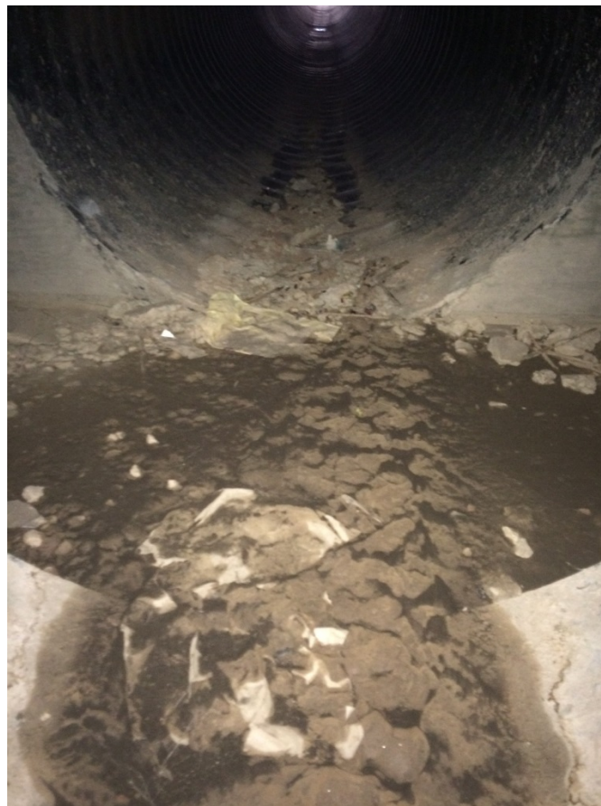
Figure 4-28: Sediment Collected in Junction Box of Station 222+00 Pipeline
