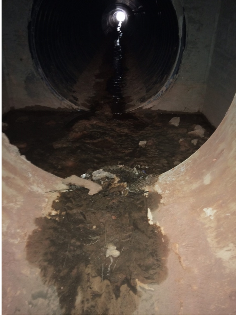
Figure 4-29: Sediment Collected in Bottom of Junction Box of Station 223+00 Pipeline
