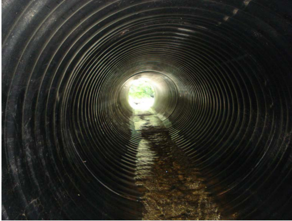
Figure 3-4: Large Internal Vertical Deflection
