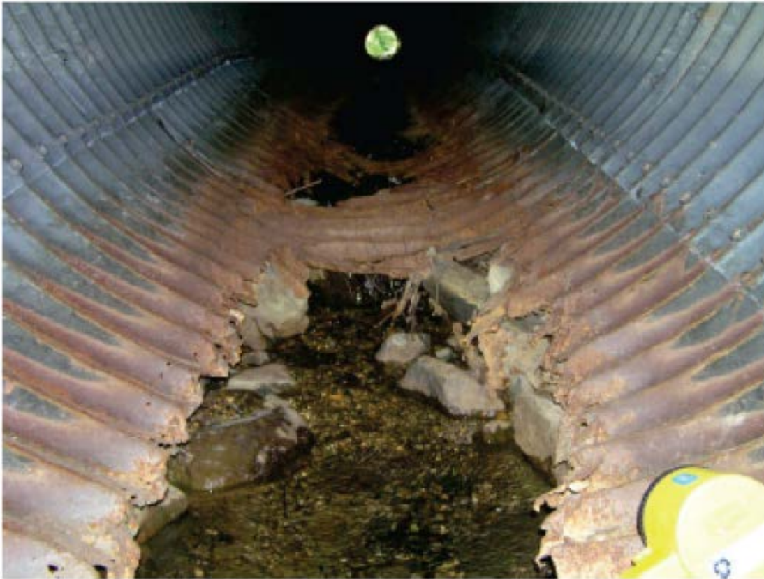
Figure 5-29: Corrosion Accelerated by Abrasion of Metal Culvert (Maher et al. 2015)
