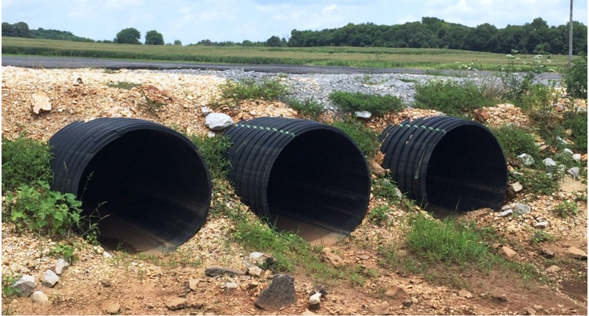
Figure 3-21: Colbert County HDPE Pipeline Side View
