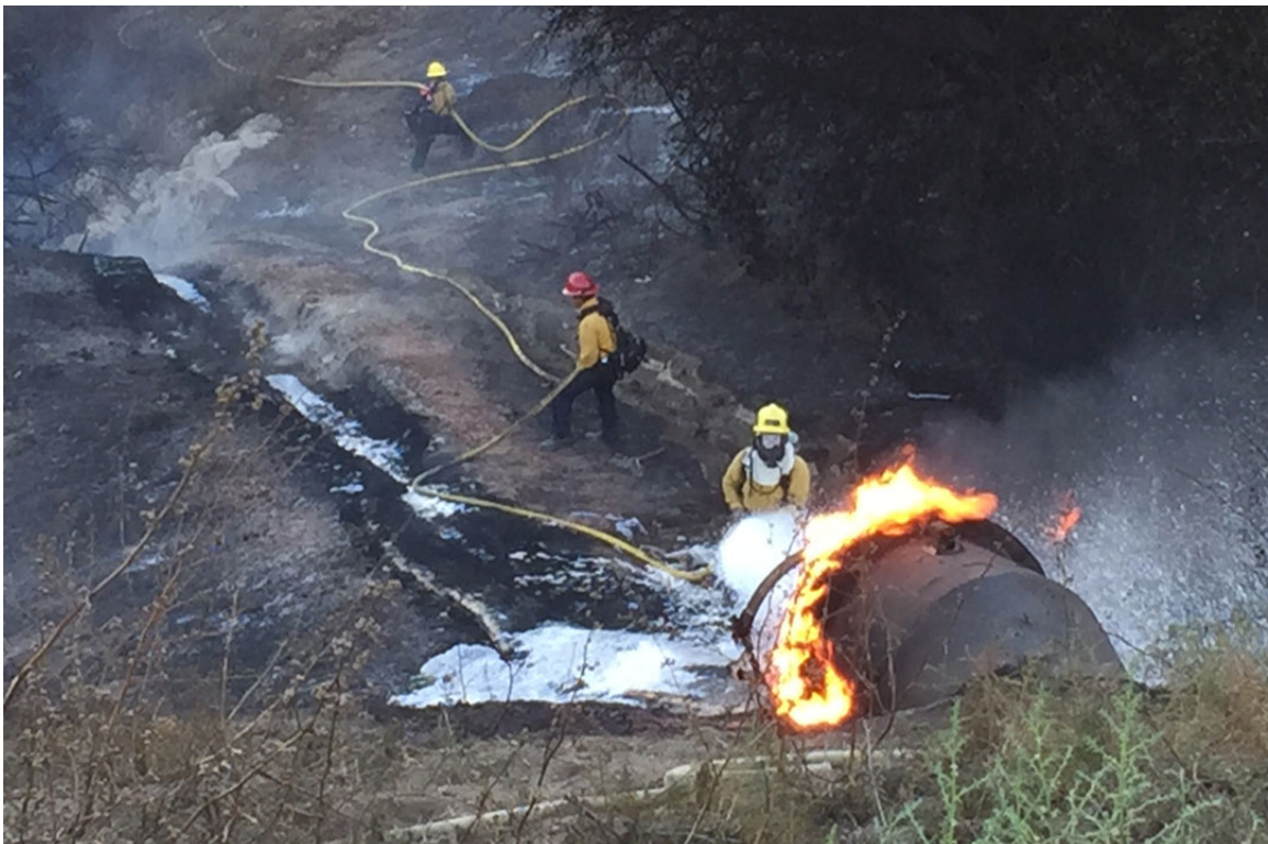
Figure 5-37: Plastic Culvert on Fire in Santa Barbara, California (Scully 2015)
