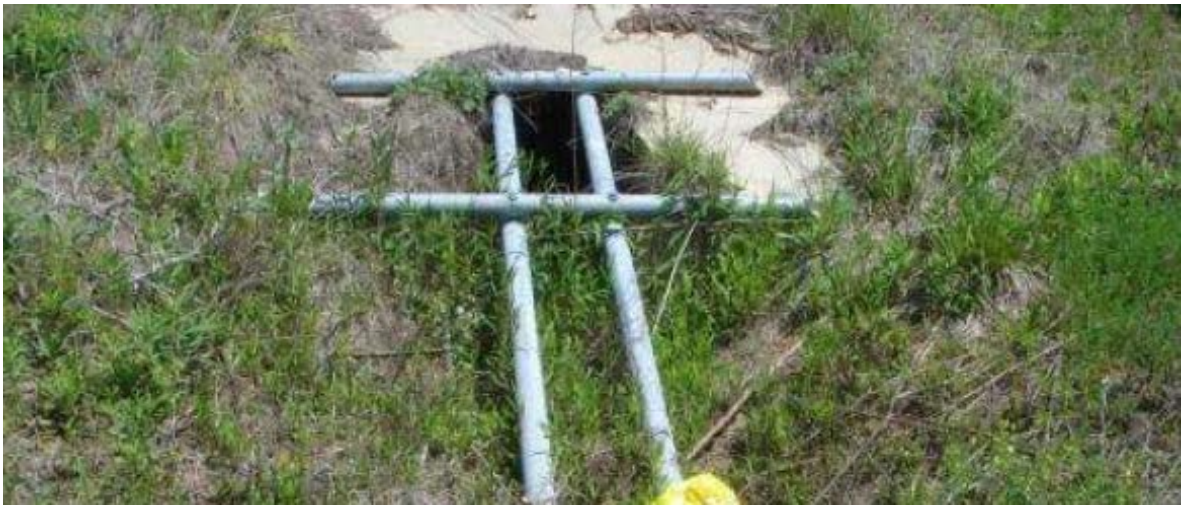
Figure 4-17: Vegetation Growth at Culverts End
