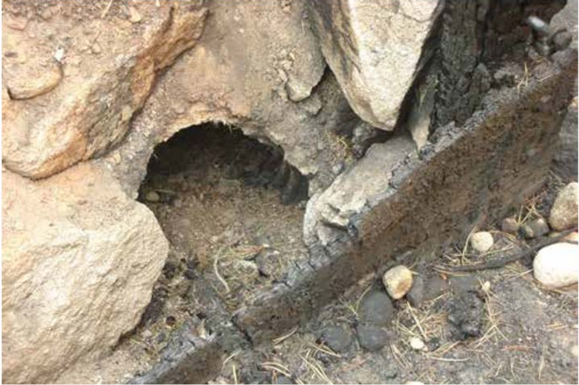
Figure 5-38: Burned High Density Polyethylene Inlet (Matthews et al. 2012)
