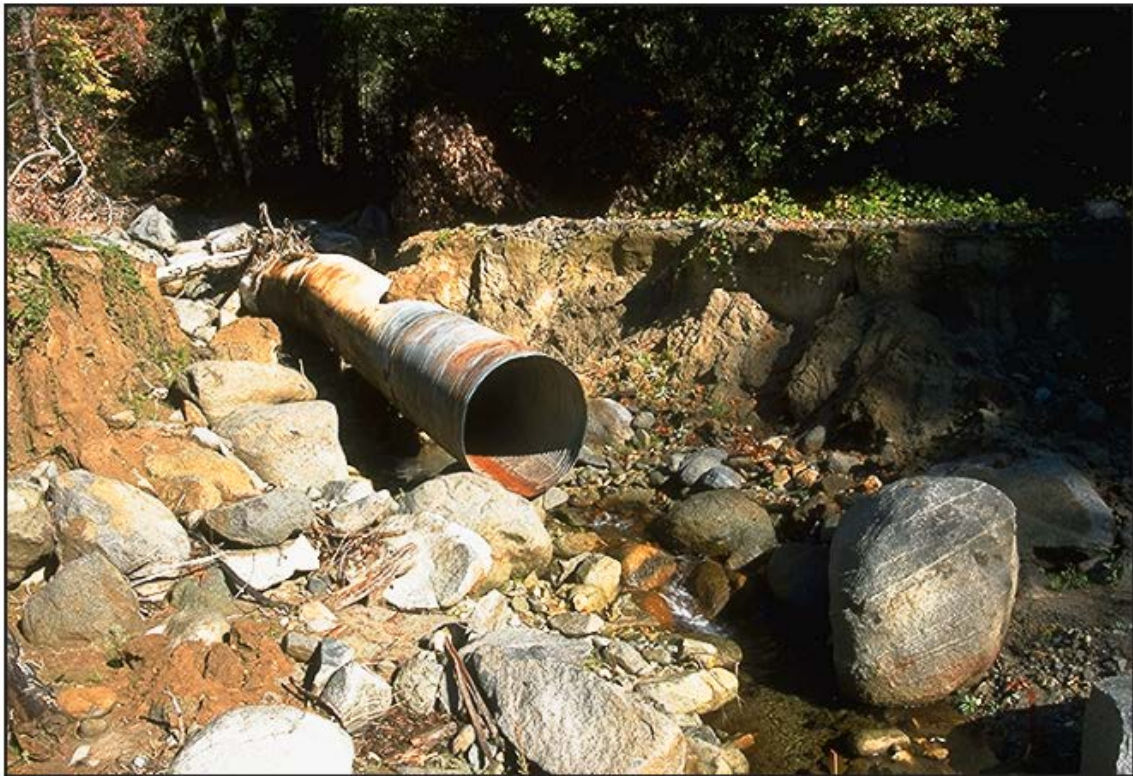
Figure 5-44: Inadequately Designed Culvert (Keller 2003)
