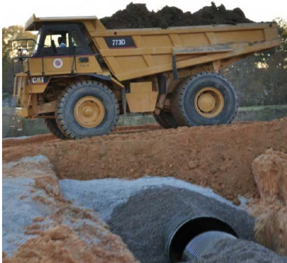
Figure 4-6: Dump Truck Driving Over Pipeline (Stuart et al. 2011)
