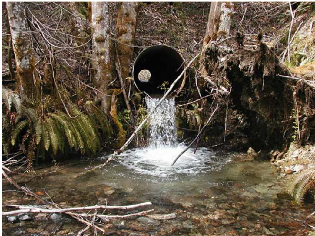
Figure 5-43: Culvert Barrier to Fish Passageway (USDA 2015)
