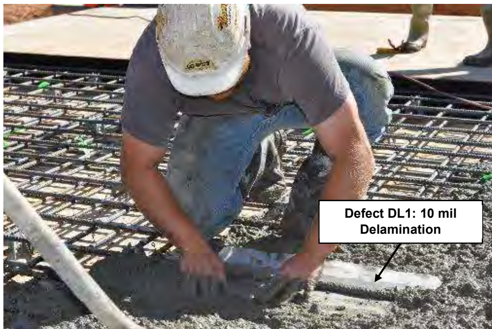
Figure 5-5: Plastic Sheetting Delamination Simulation in Test Bridge
