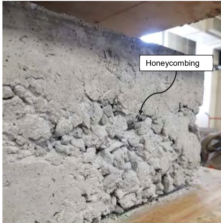
Figure 2-3: Honeycombing in a Concrete Slab
