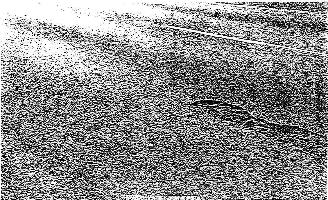
Figure 2.2. I-65 Deck Surface Spall
