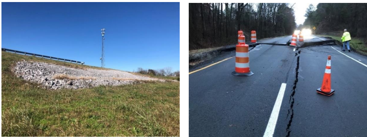
Figure 2-1: (Left) A repaired slope failure in an embankment section of SR-5 in Perry County and (right) cracking in the southbound lanes of US-231 near Laceys Spring following a large landslide in 2020.
