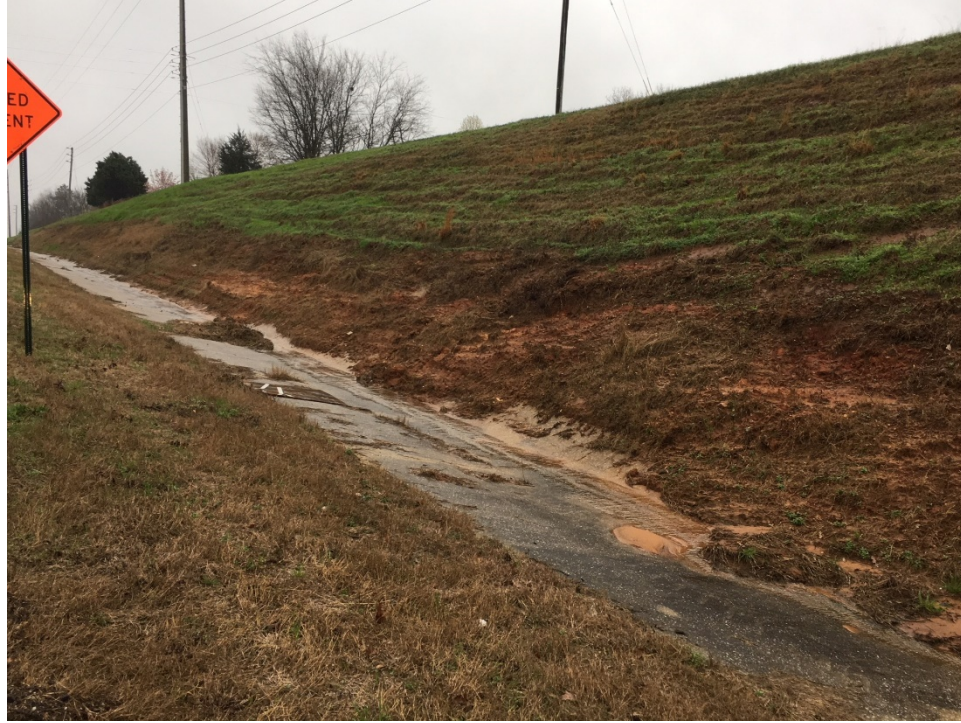
Figure 2-5. Shallow slope failures caused by rutting from mowing activities along Highway 69 near mile post 137.7 (photo provided by Jacob Hodnett, ALDOT).
