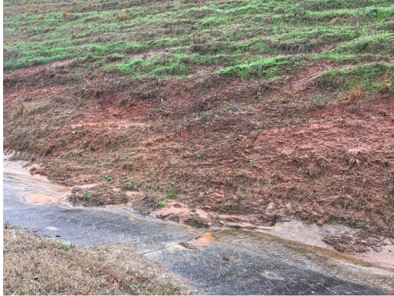
Figure 3-6. Shallow slope failures caused by rutting from mowing activities along Highway 69 near mile post 137.7 (photo provided by Jacob Hodnett, ALDOT).
