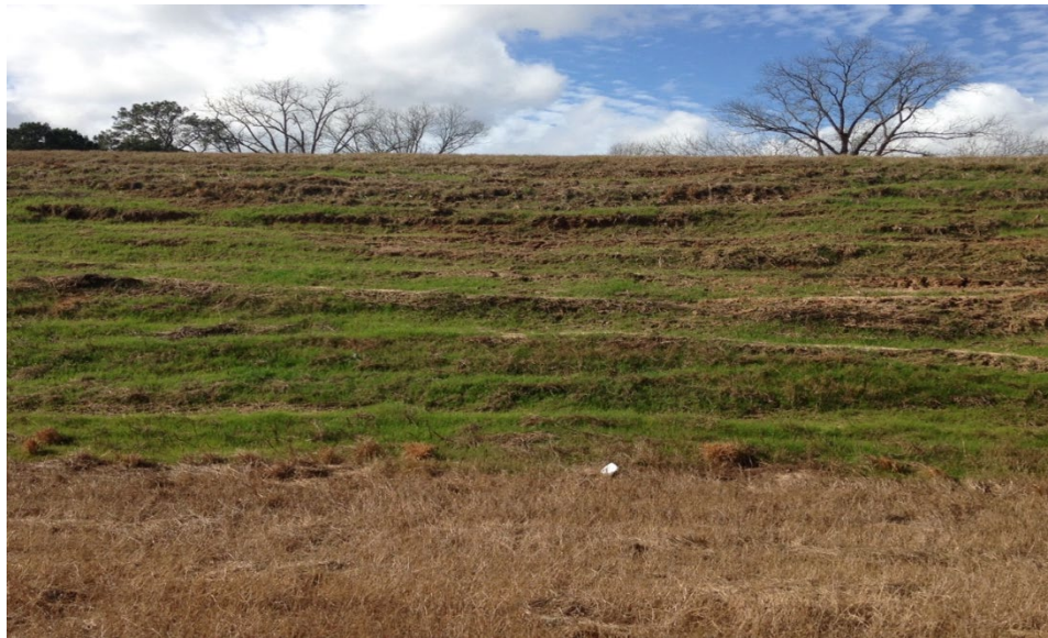
Figure 3-5. Rutting along the face of a slope due to mowing activities (photo provided by Jacob Hodnett, ALDOT).
