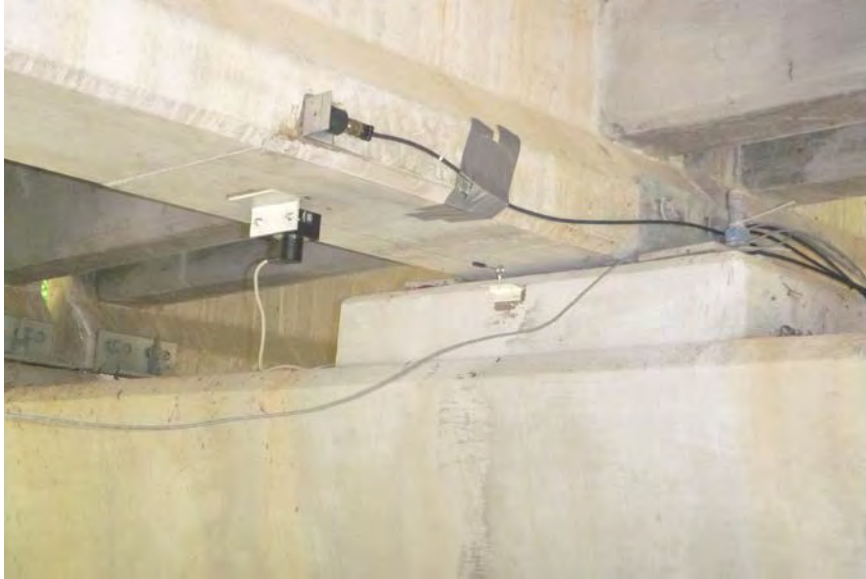
Figure 4-11 Instrumentation and Cabling
