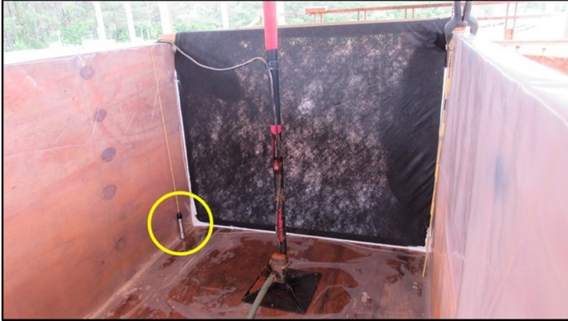
Figure 7. Upstream water level logger installation location.
