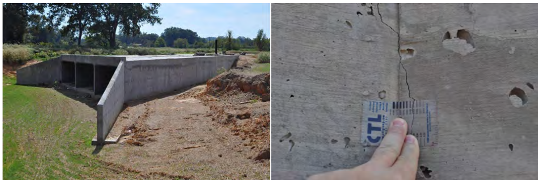
Figure 1-2. Culvert distress near Centerville, AL
