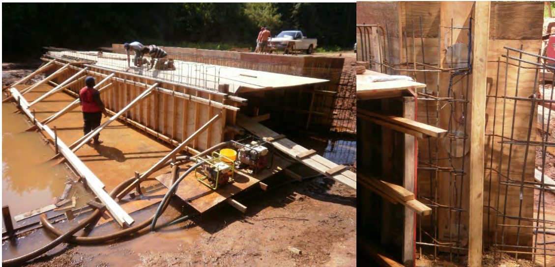
Figure 4-10. Workers construct formwork for southern end of culvert and formwork for embedded pressure cells
