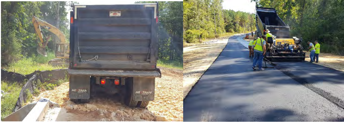
Figure 4-17. 40 ton truck placed near tab and culvert in process of being paved
