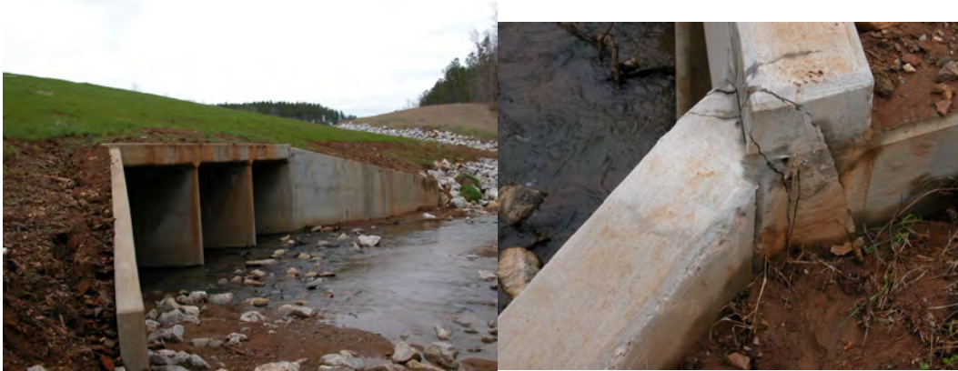
Figure 1-1. Culvert distress on AL 49 near Dadeville, AL
