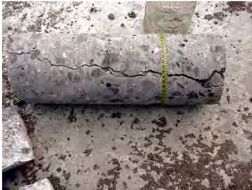
Figure 2-15: Core from footing exposed to thermal shock (Gajda and Alsamsam 2006)
