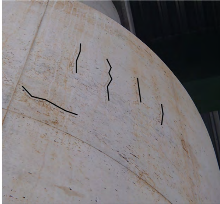
Figure 5-19: Scottsboro pedestal close-up of cracks observed at top of pedestal (unreachable)
