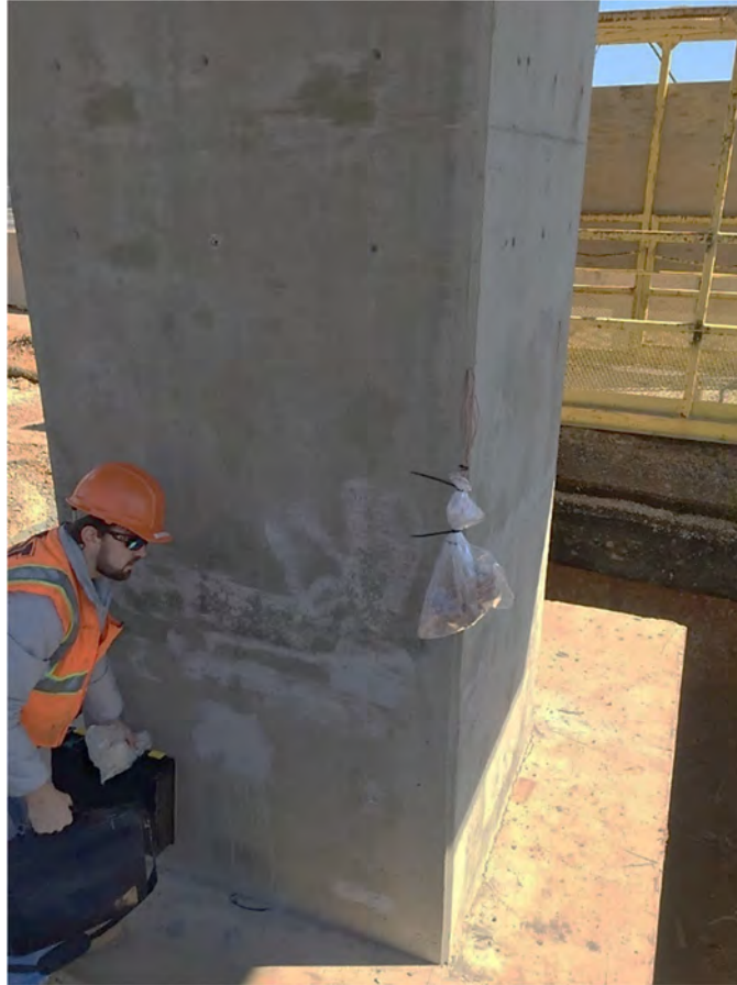
Figure 5-29: Birmingham column post construction with sensor lead wires visible
