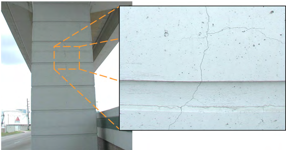
Figure 2-6: Thermal cracking in a Texas bridge element (Photo courtesy of Dr. J.C. Liu)
