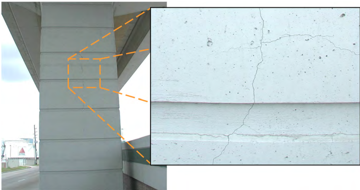
Figure 1-1: Thermal cracking of a bridge column in Texas (Photo Courtesy of Dr. J.C. Liu)
