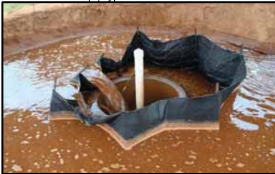
(c) hexagonal configuration failure
