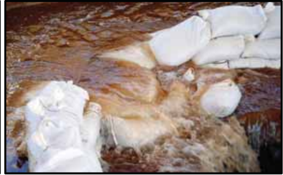
(b) ALDOT standard installation failure
