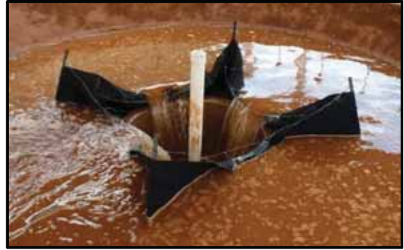
(b) typical installation failure
