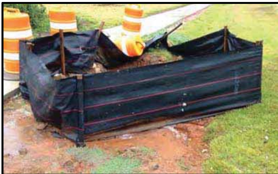
(e) improper trenching of installation
