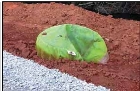
(b) damaged installation
