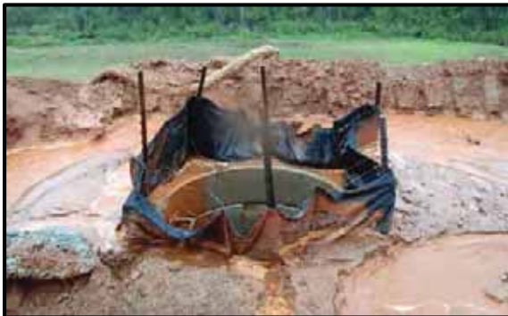
(c) structural failure and flow bypass
