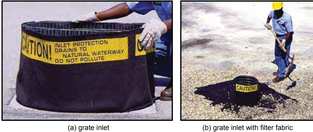
Figure 2.22 Ultra-Basin Guard Installations(UltraTech International 2014).
