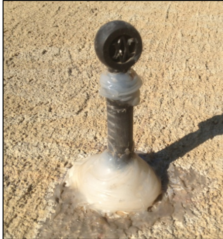
Figure 6-4: Plastic tube with rubber plug installed in concrete
