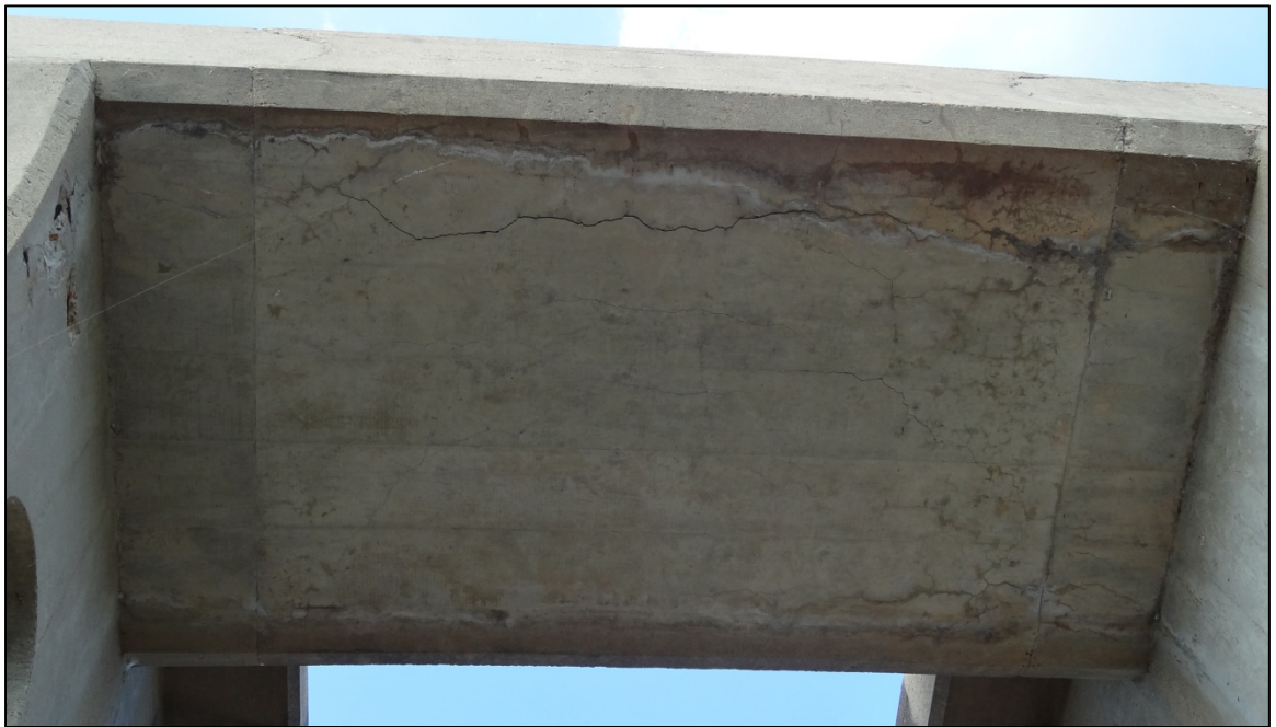
Figure 8-11: Examples of possible ASR in span 4
