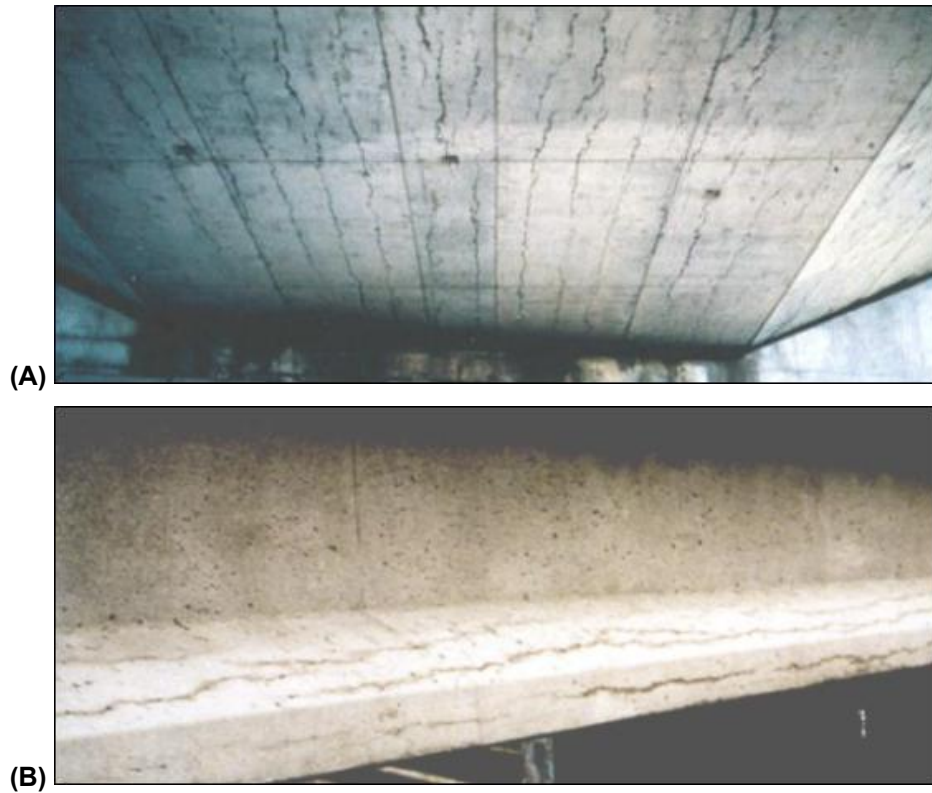
Figure 2-4: Longitudinal cracking due to ASR in (A) a bridge deck soffit and (B) a precast, reinforced concrete beam (Fournier et al. 2010)
