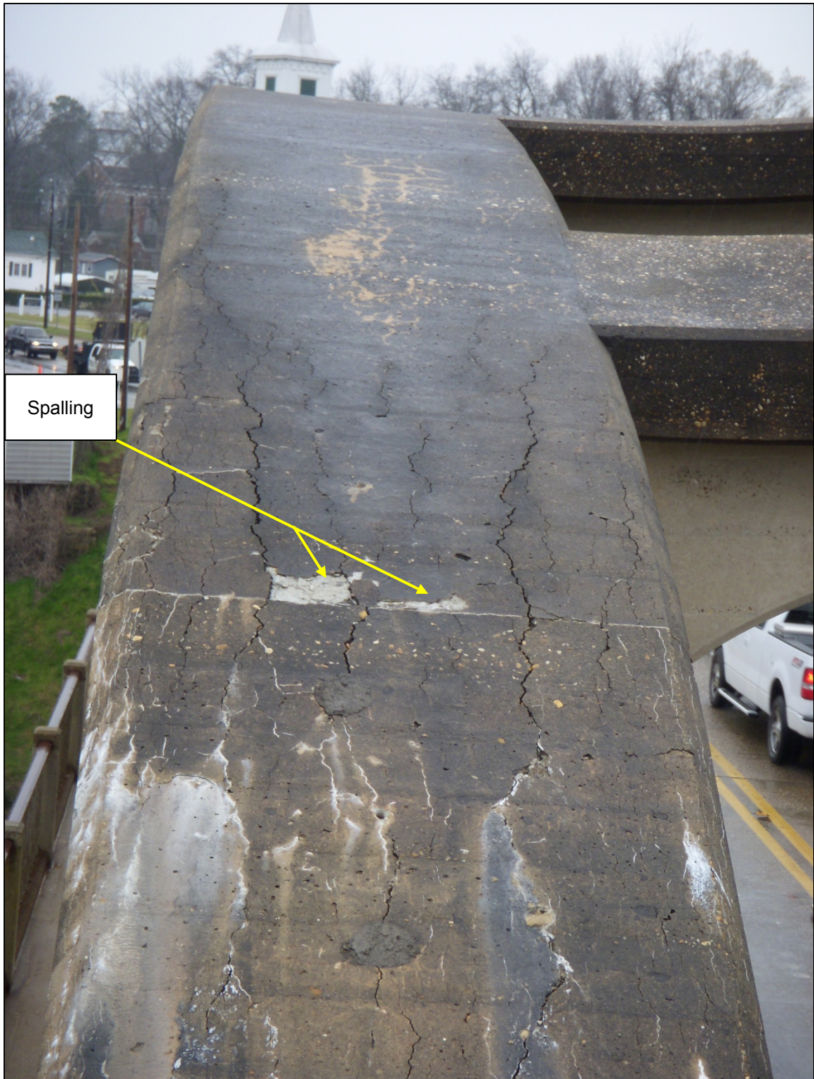
Figure 3-18: Closer view of longitudinal cracking and spalling on span 5 south on 3/11/08
