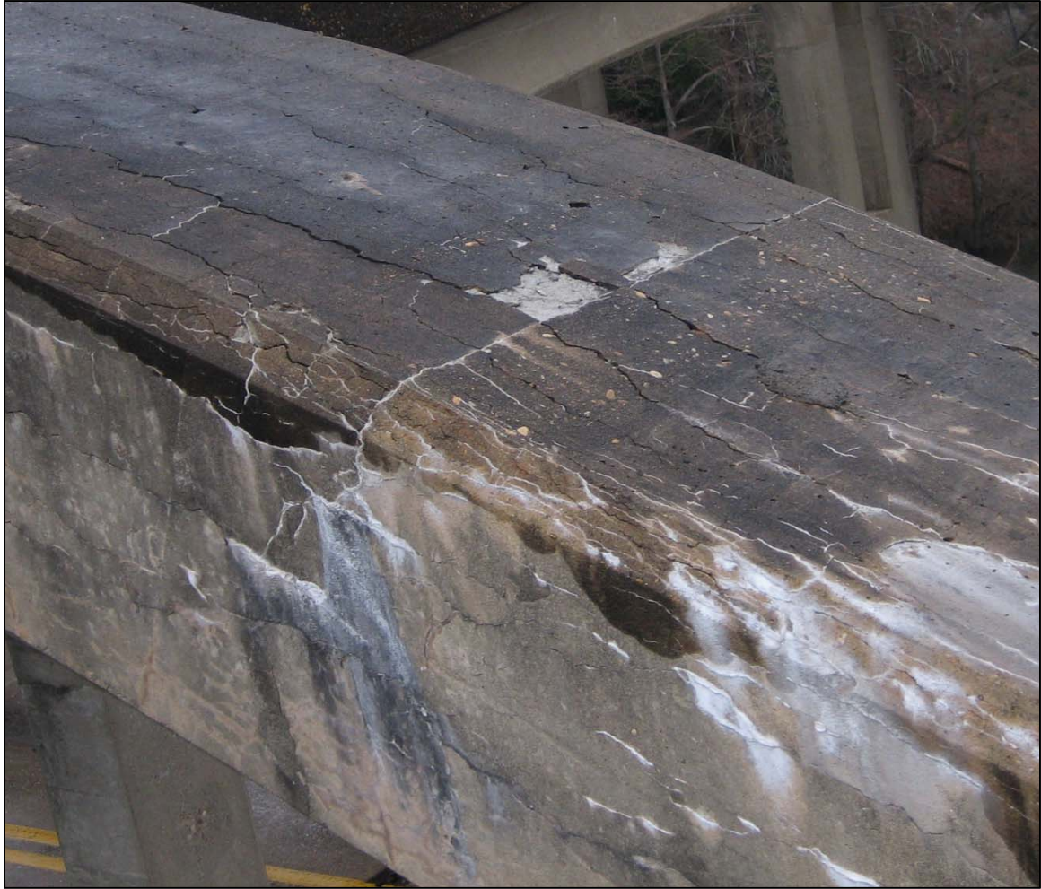
Figure 1-2: Surface deposits and ASR-induced cracking on 3/11/08
