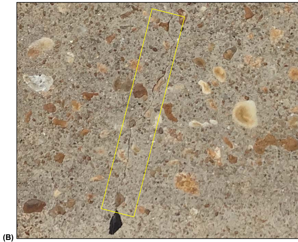
Figure 7-18: Crack widening on span 5 – south arch, (A) November 2010 and (B) August 2013
