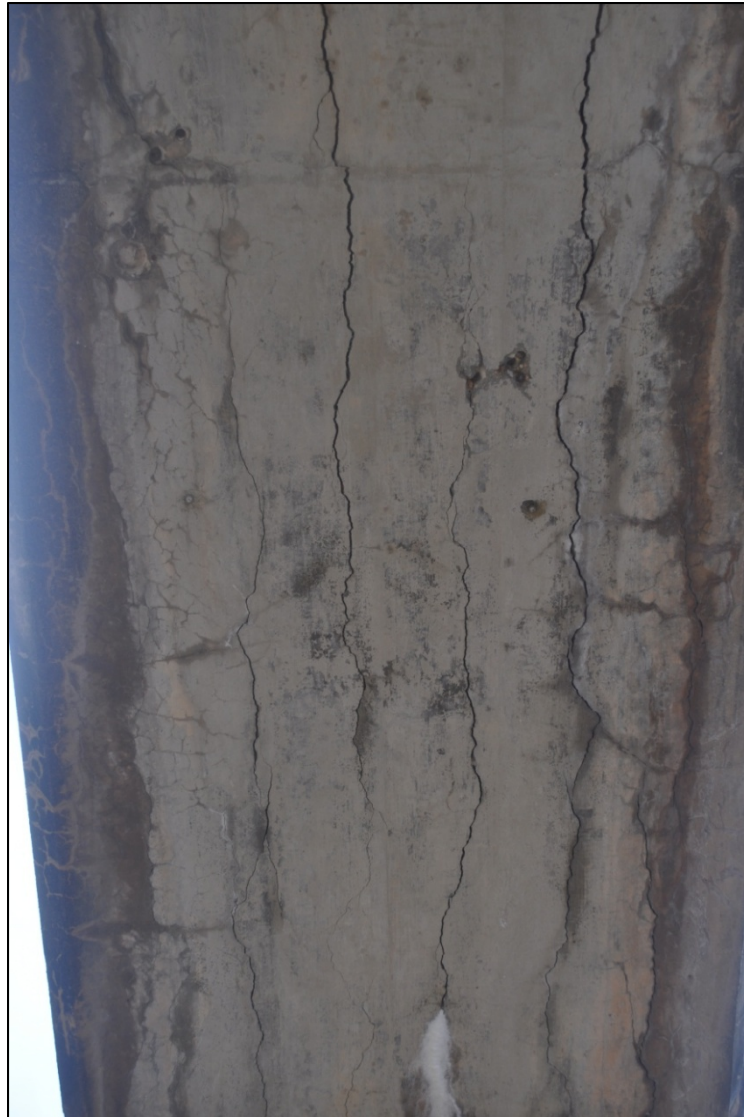
Figure 3-21: Cracking and surface discoloration on the bottom of an arch
