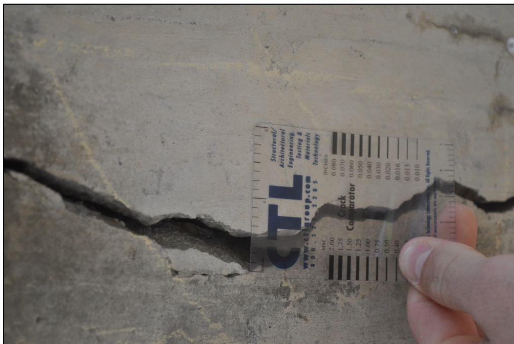
Figure 3-20: Crack width close to 1/2 inch
