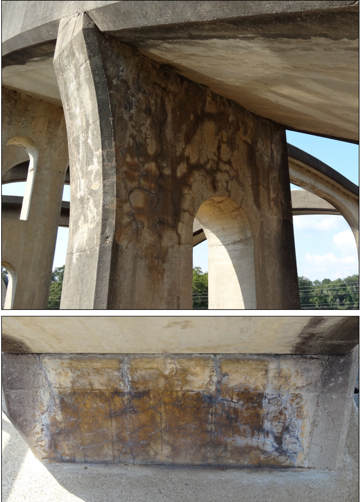
Figure 8-10: Examples of possible ASR in span 3
