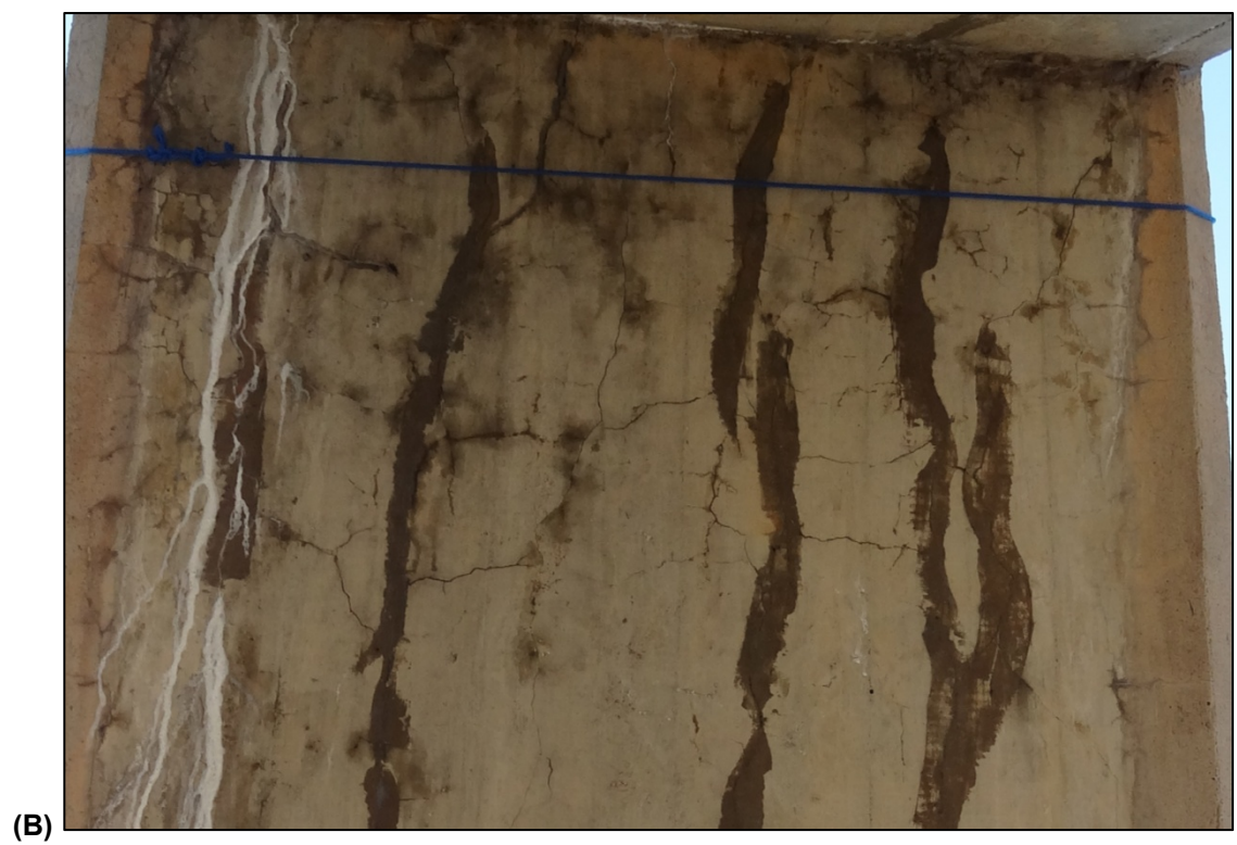
Figure 7-14: Additional cracking in span 5 – north arch, (A) November 2010 and (B) August 2013
