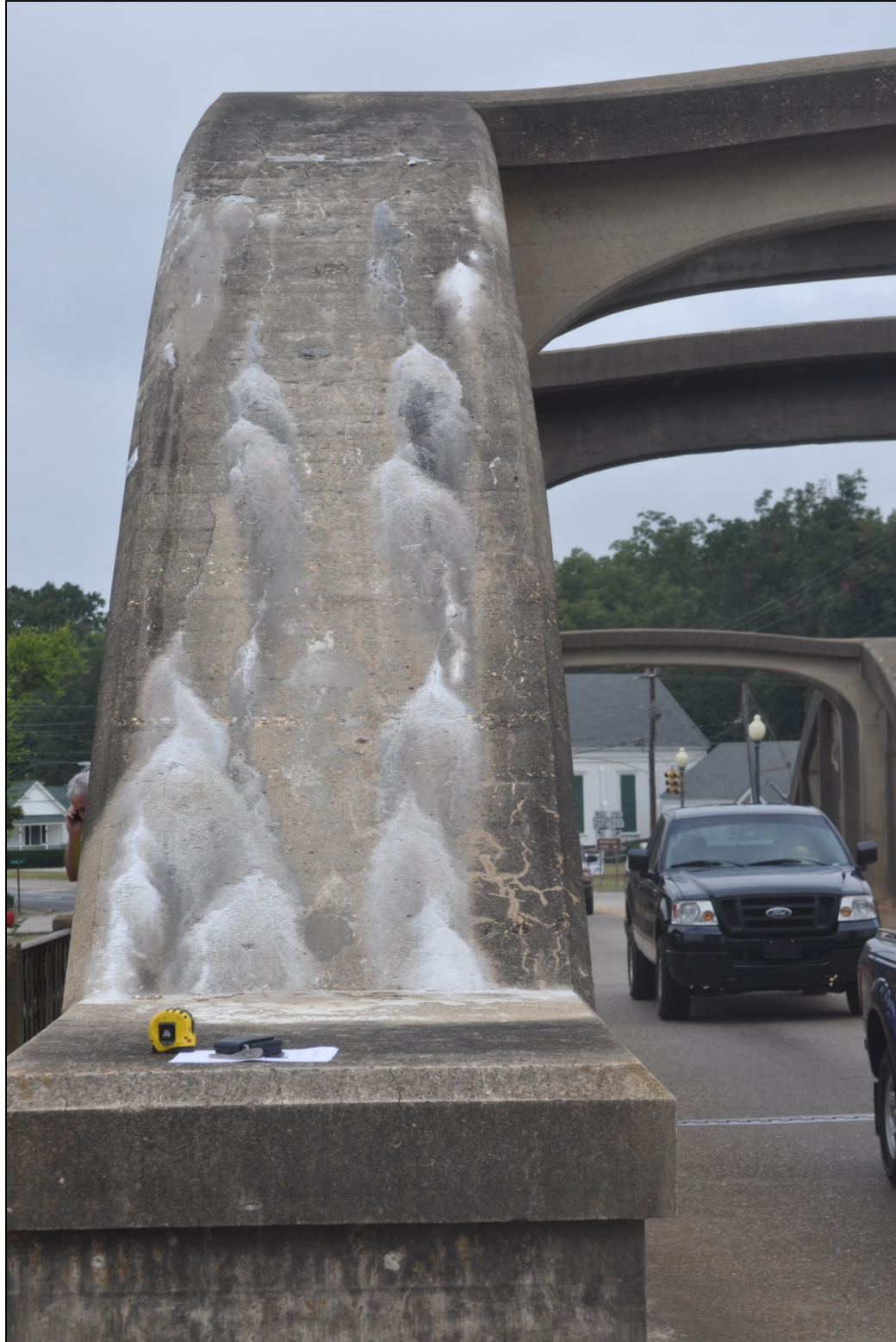
Figure 3-17: Distress with surface deposits of efflorescence and alkali-silica gel on the eastern side of span 5 south
