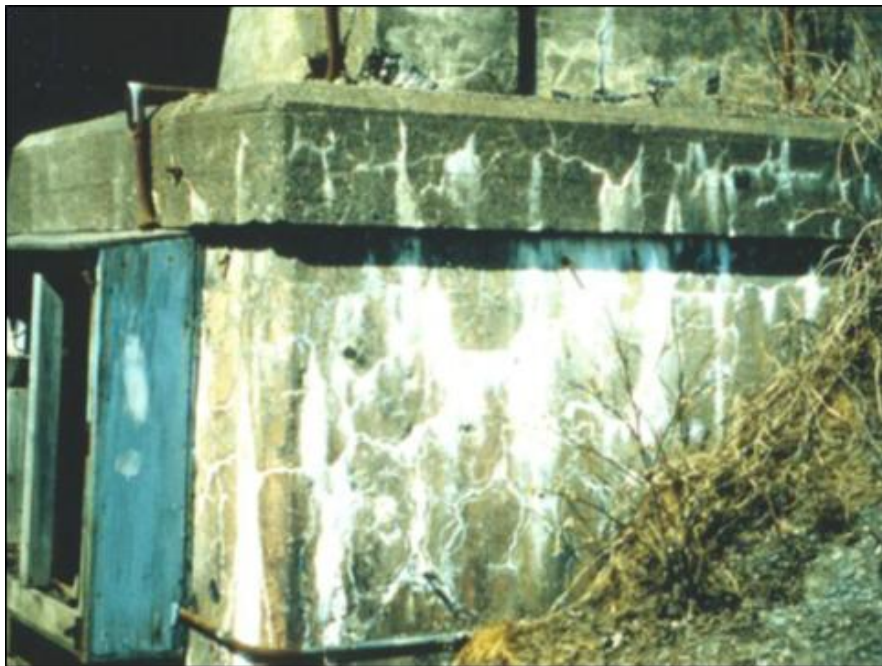
Figure 2-5: Efflorescence and exudations of alkali-silica gel on a foundation (Fournier et al. 2010)
