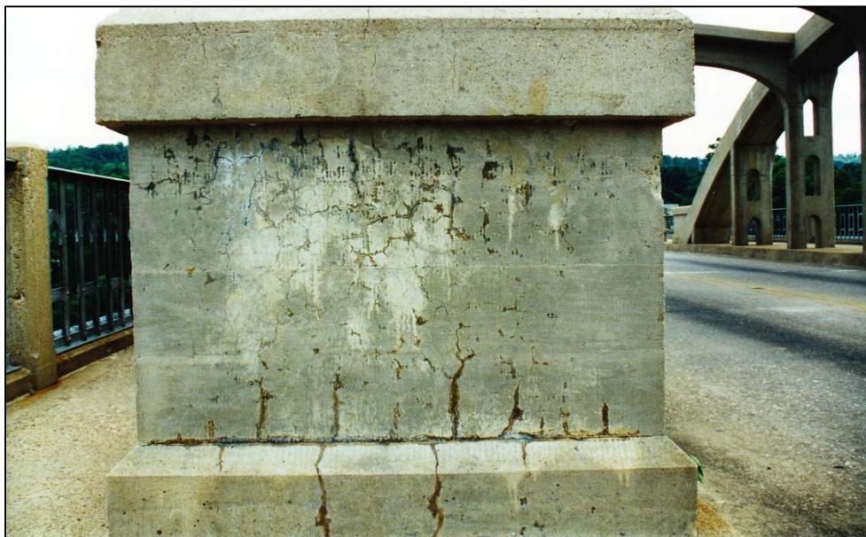
Figure 3-23: Map-cracking on an abutment of span 5
