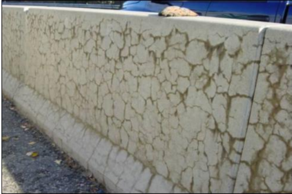
Figure 2-3: Severe map-cracking and surface discoloration on a road barrier (Fournier et al. 2010)
