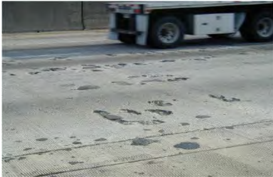
Figure 2.1 Typical Deck Deterioration (Umphrey 2006)
