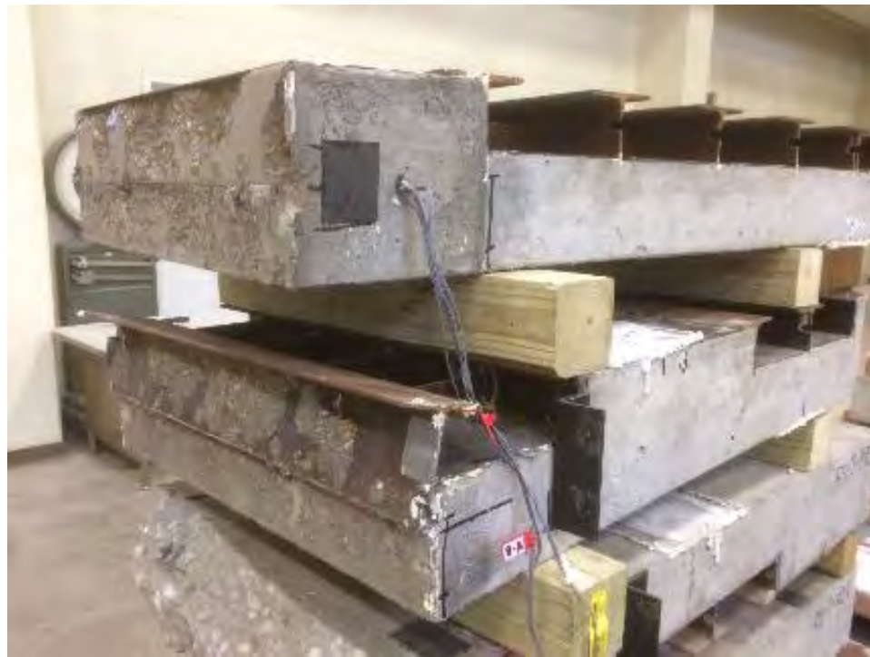
Figure 5.50 Separated (and Inverted) Deck Panels (R-NEG-F)
