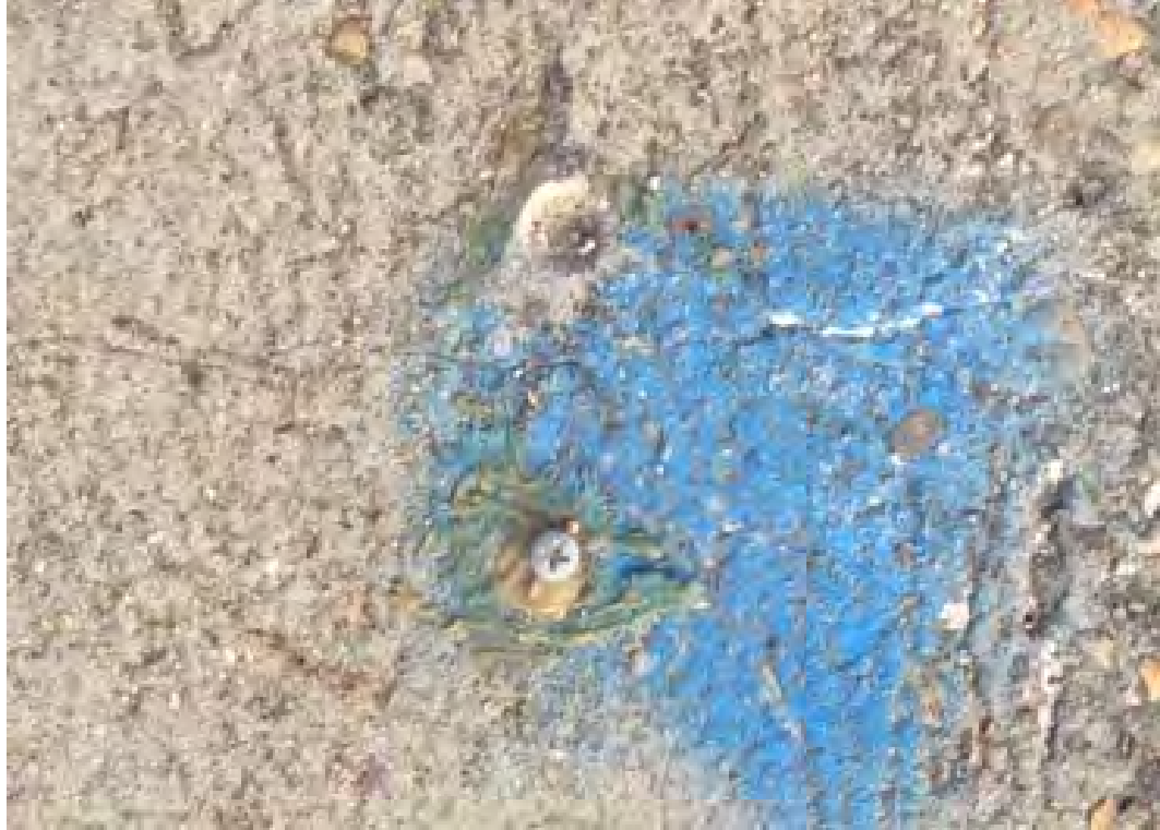
Figure 5.22 Transducer Mount Damaged by Traffic
