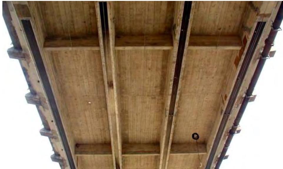
Figure 2.4 EB FRP Laminate Retrofit of the War Memorial Bridge (Carmichael and Barnes 2005)
