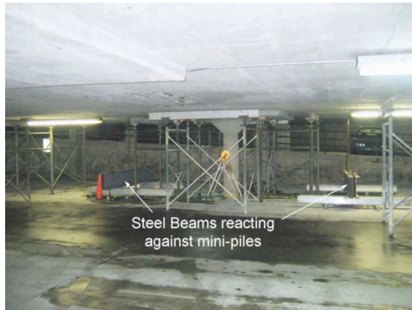
Figure 2.13 Reaction Beams on Mini-Piles to Load Decks Above (Tumialan, Vatovec, and Kelley 2007).
