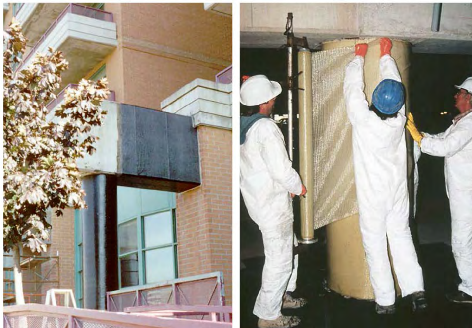
Figure 2.3 FRP Fabric Wraps of Beam (Left) and Column (Right) (Sheikh and Homam 2004)
