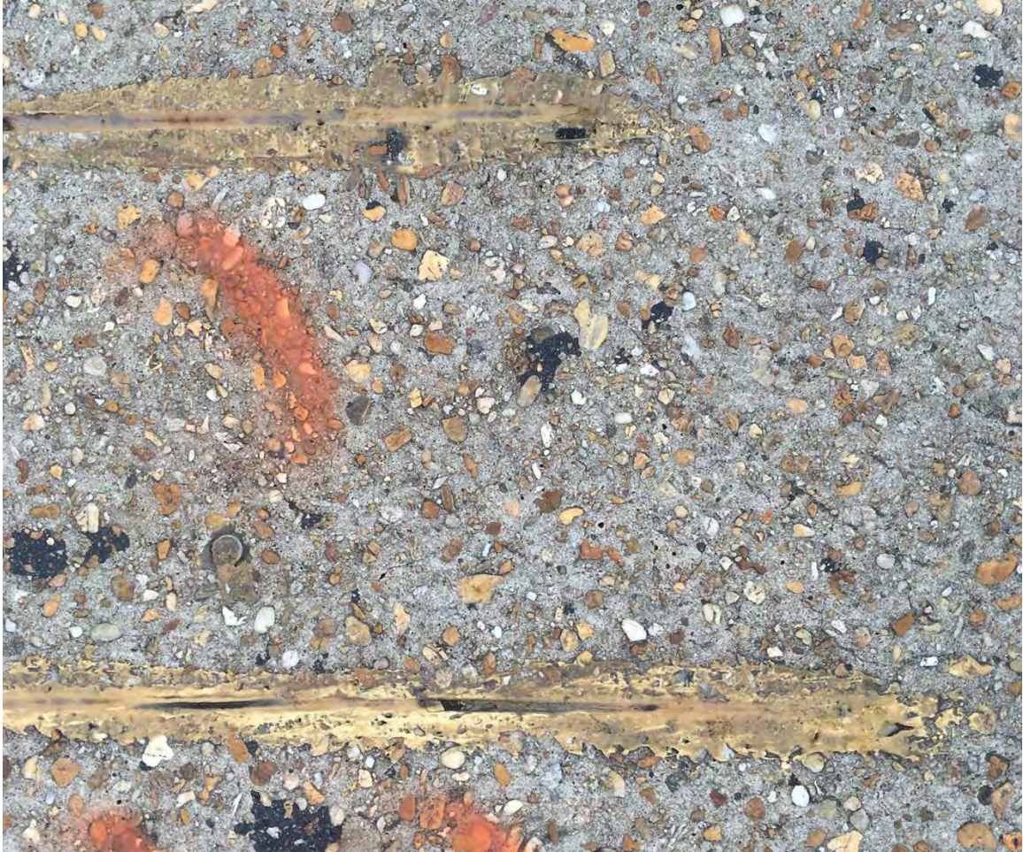
Figure 6.18 Degradation of Epoxy Near Ends of Strips
