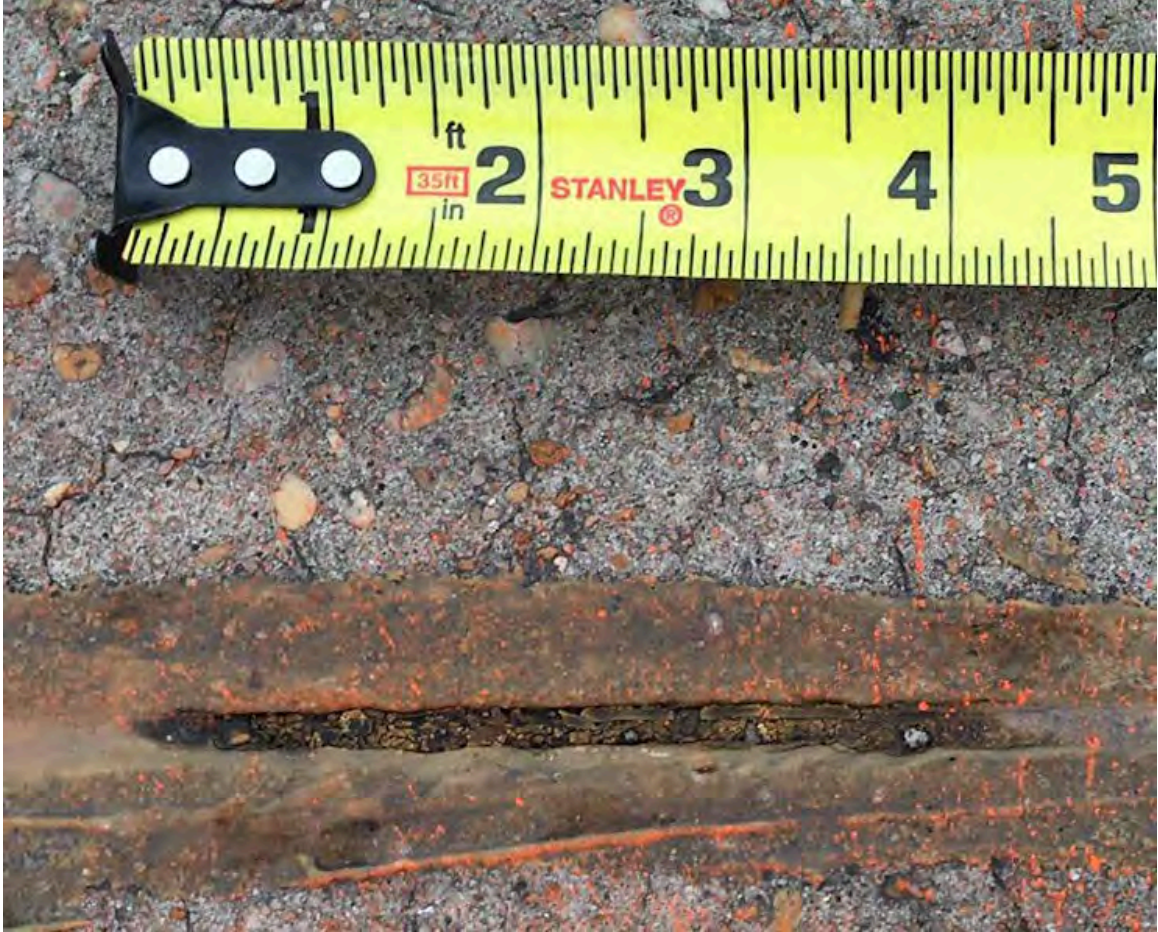
Figure 6.17 Typical Area of Epoxy Degradation
