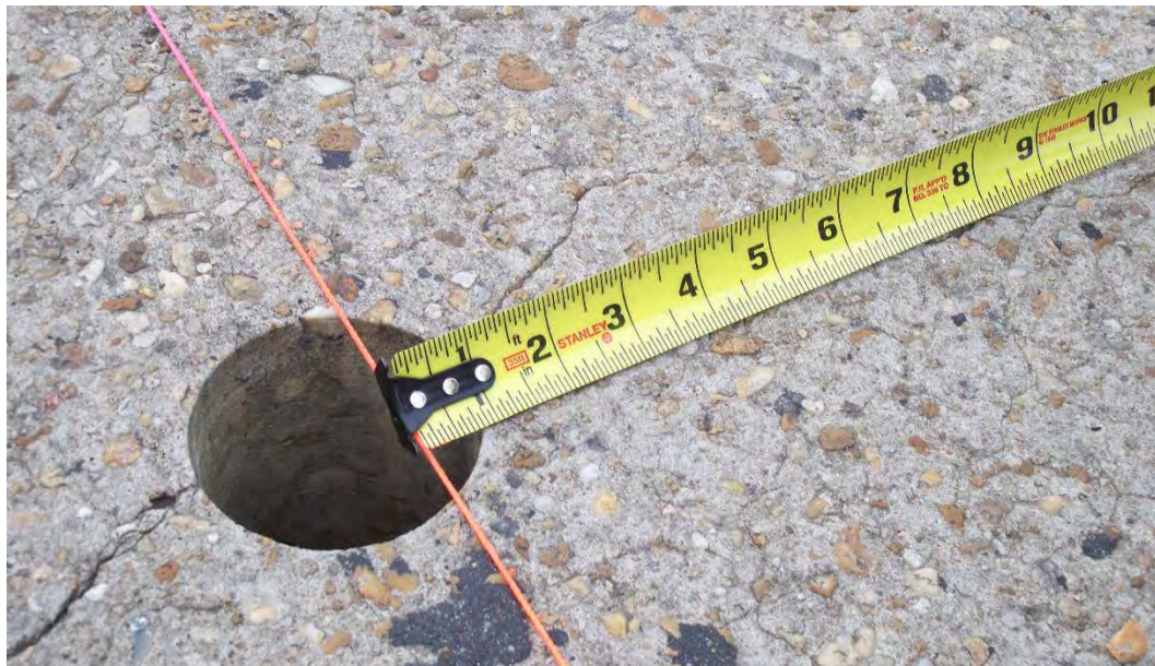
Figure 4.13 Core and FRP Strip Location Conflict
