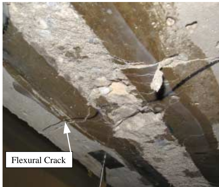
Figure 5.4 Concrete Substrate after FRP Debonding
