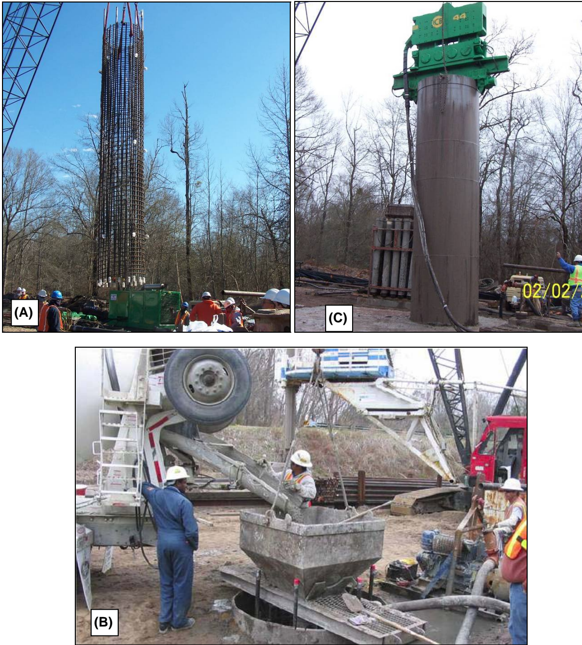
Figure 1: Construction of shafts: (A) Reinforcement cage, (B) Tremie placement of concrete, (C) Removal of permanent casing
