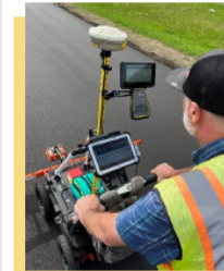
Collected data is shown on the equipment's screen, allowing for compaction adjustments in real time.
