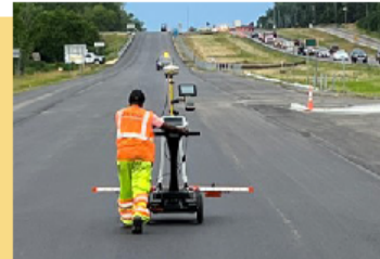
By rolling a DPS unit over the newly paved roadway, crews measured the pavement's density in real time.
