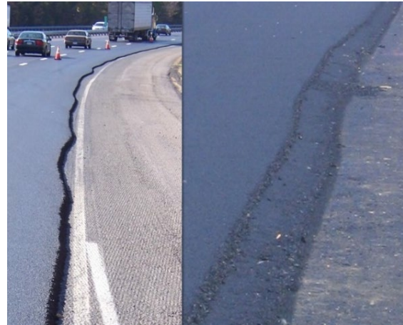
Figure 7. Examples of Uneven Unconfined Joint Edge (Butt & Notched-wedge Joints).
