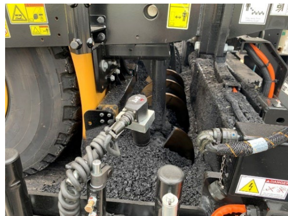
Figure 8. Example of the Proper Head of Material in the Auger Chamber, where about half of the Auger is Exposed.
