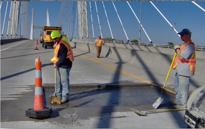
Effective removal of concrete to be replaced Then clean and patch well
