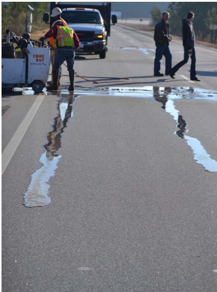
Figure 5.5 Water Pooling in Ruts (Trench 2)
