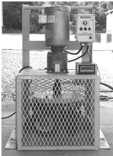
Figure 24. Protective Wire Mesh
