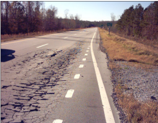
Advanced fatigue cracking in structural Test Section N1
