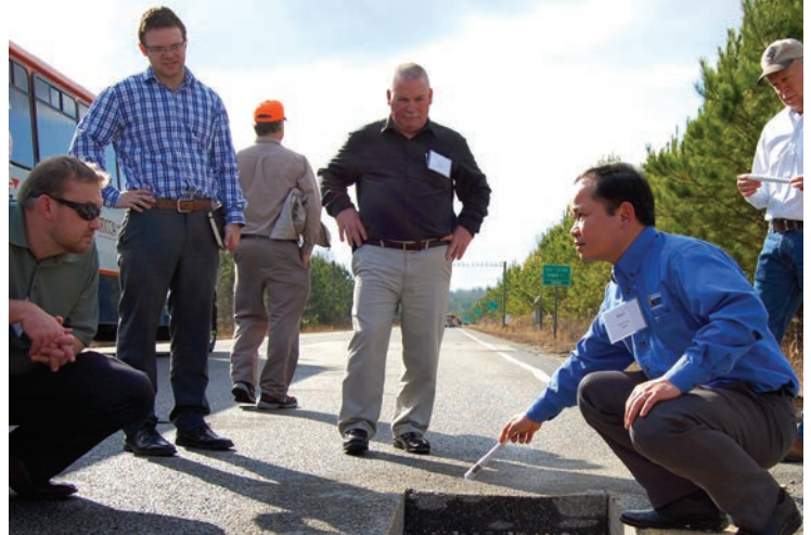
Nam Tran discusses the interlayer bond and points out cracks that can be seen in the trench.
