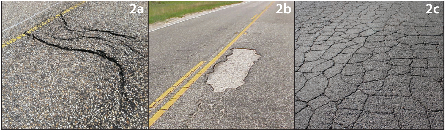
Figure 2: Common distresses associated with poor bonding of layers include slippage cracks, delamination, and alligator cracking, as shown in 2a, 2b, and 2c, respectively.
